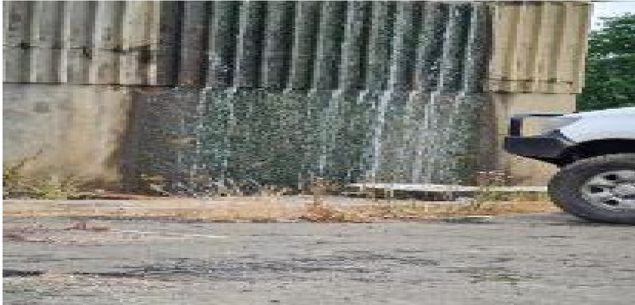
Figure 4.17: Water loss due to overflow from flocculation channels daily
