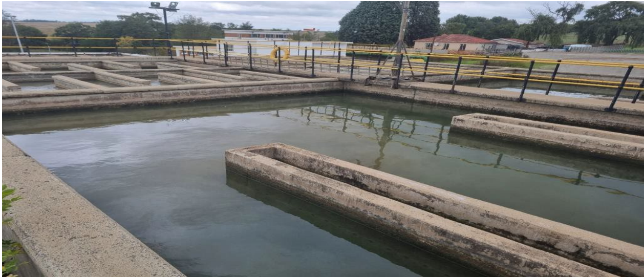
Figure 4.19: Standerton Water Treatment Works
