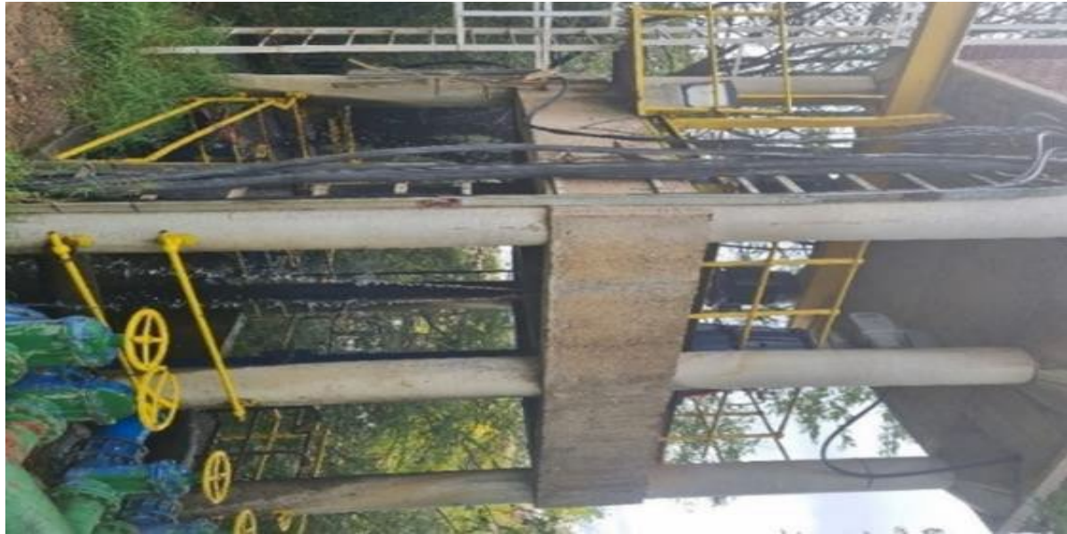
Figure 4.1: Raw water pumps 1 and 2 closer to Vaal River
