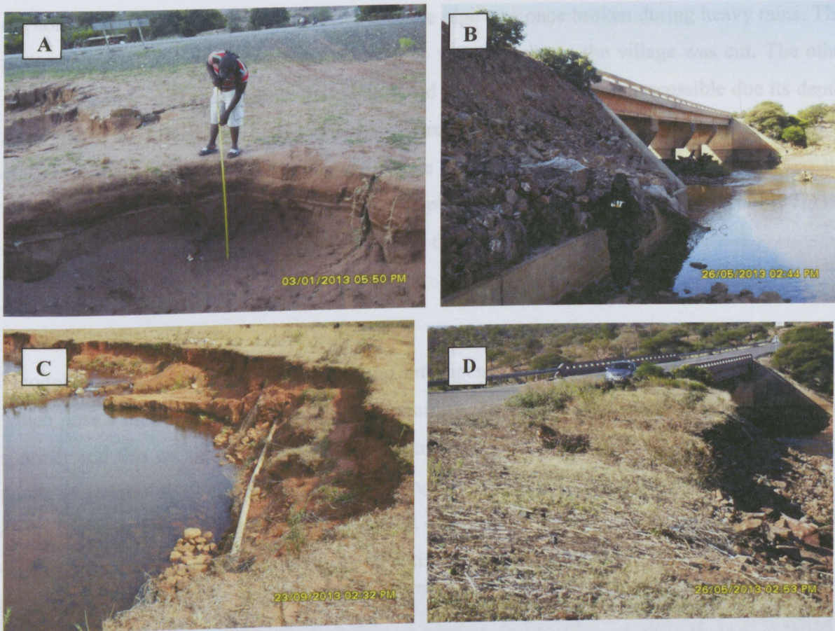
Figure 4.11 Exposed bridge foundation and water pipe line
