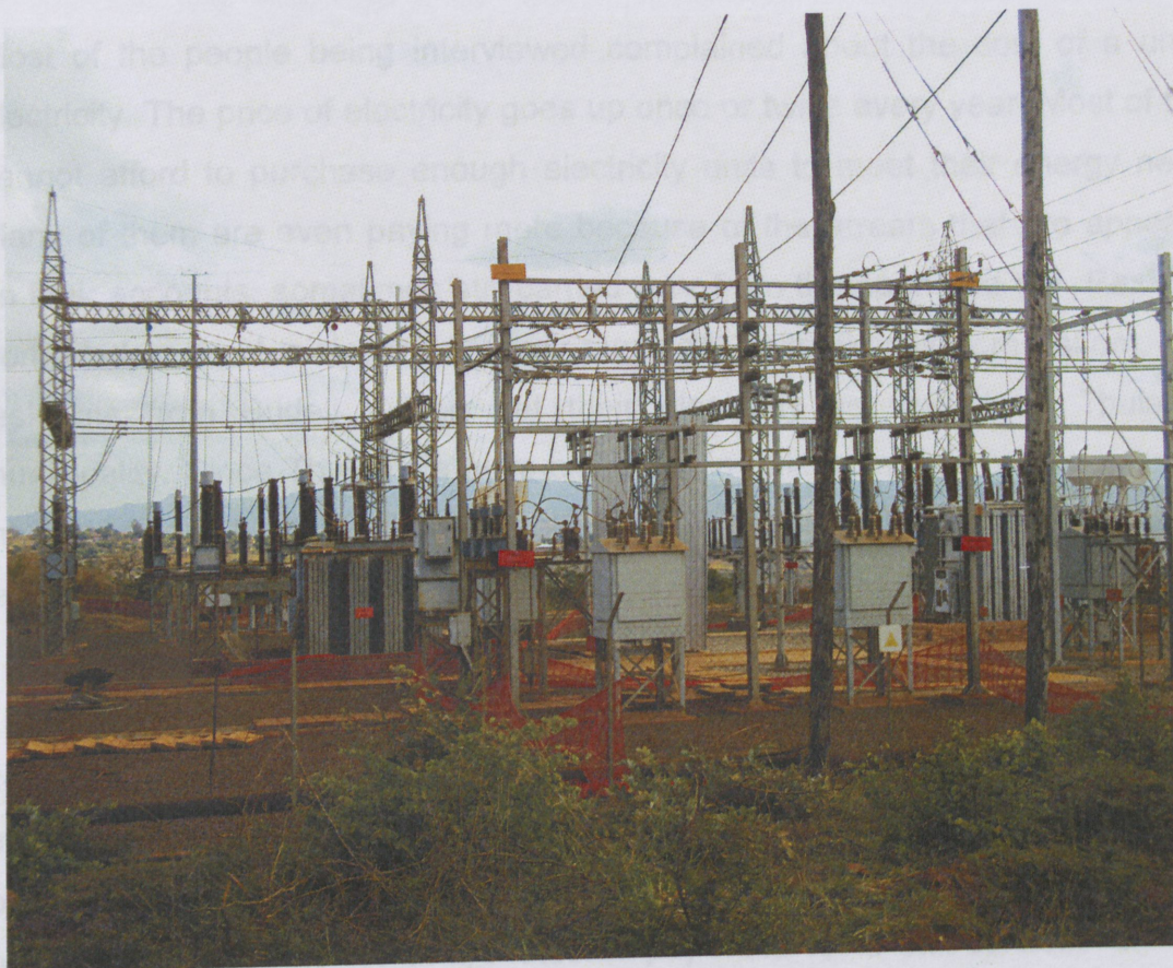
Picture 4.6: Main power station situated in Tshikweta village
