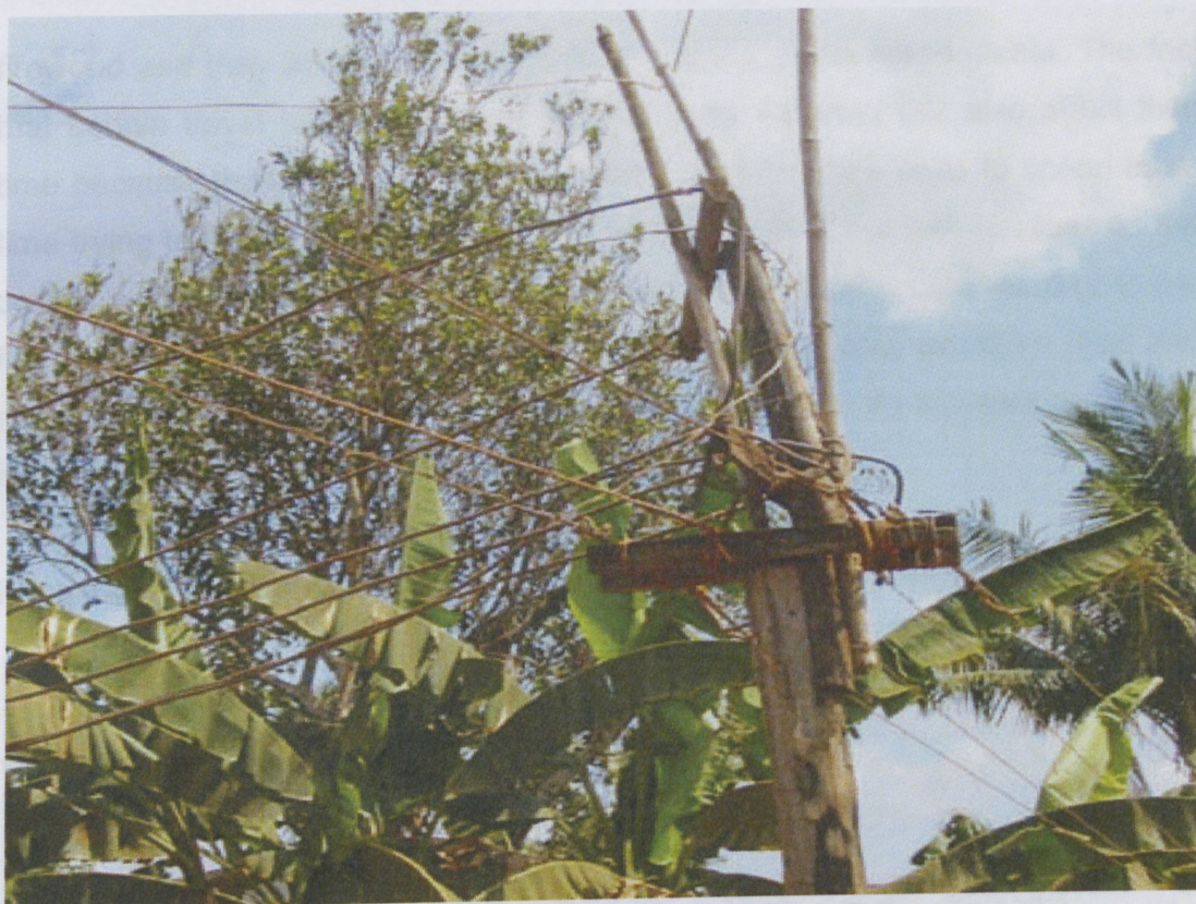
Picture 4.1: Poor maintenance of electricity supply system in Mukumbani village (Source survey data: 2011)
