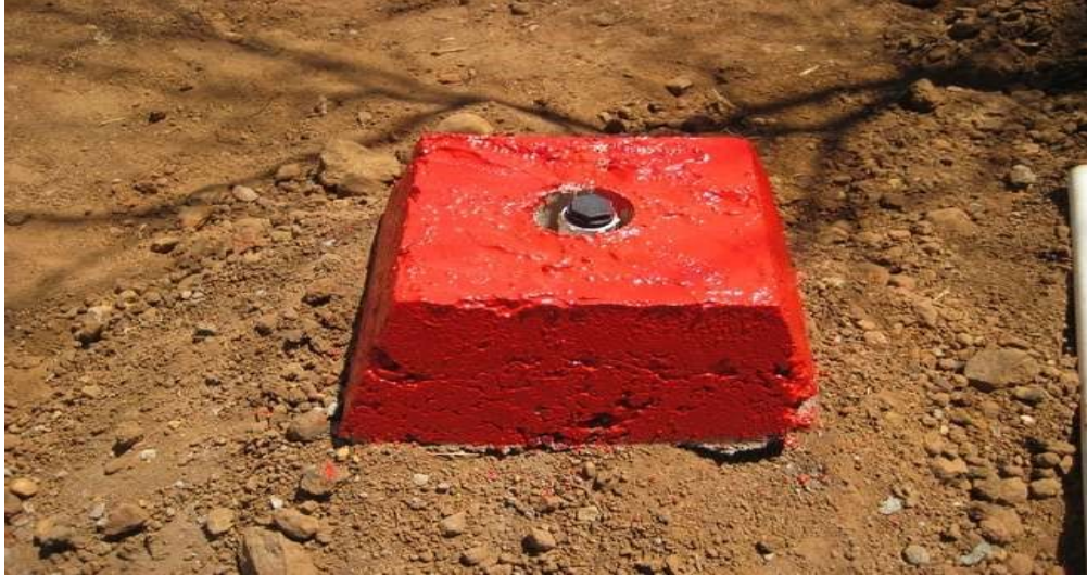
Plate 3.1: Pictorial image of an installed LFG monitoring probe installed in the landfill
