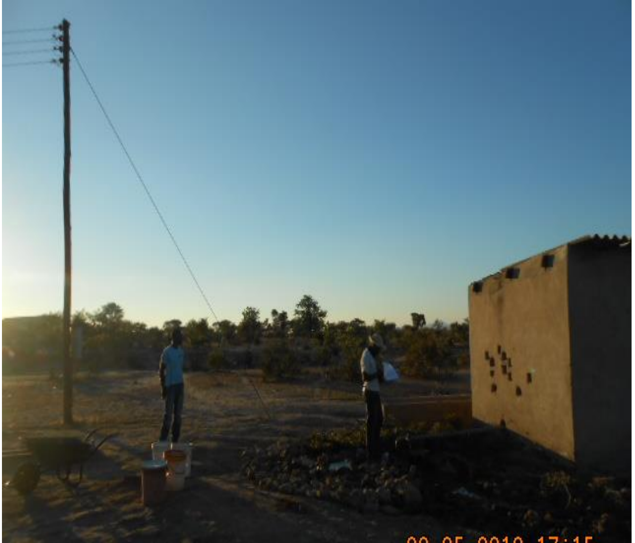
Figure 4.1 Electrified pump providing purified household water to residents in ward 12
