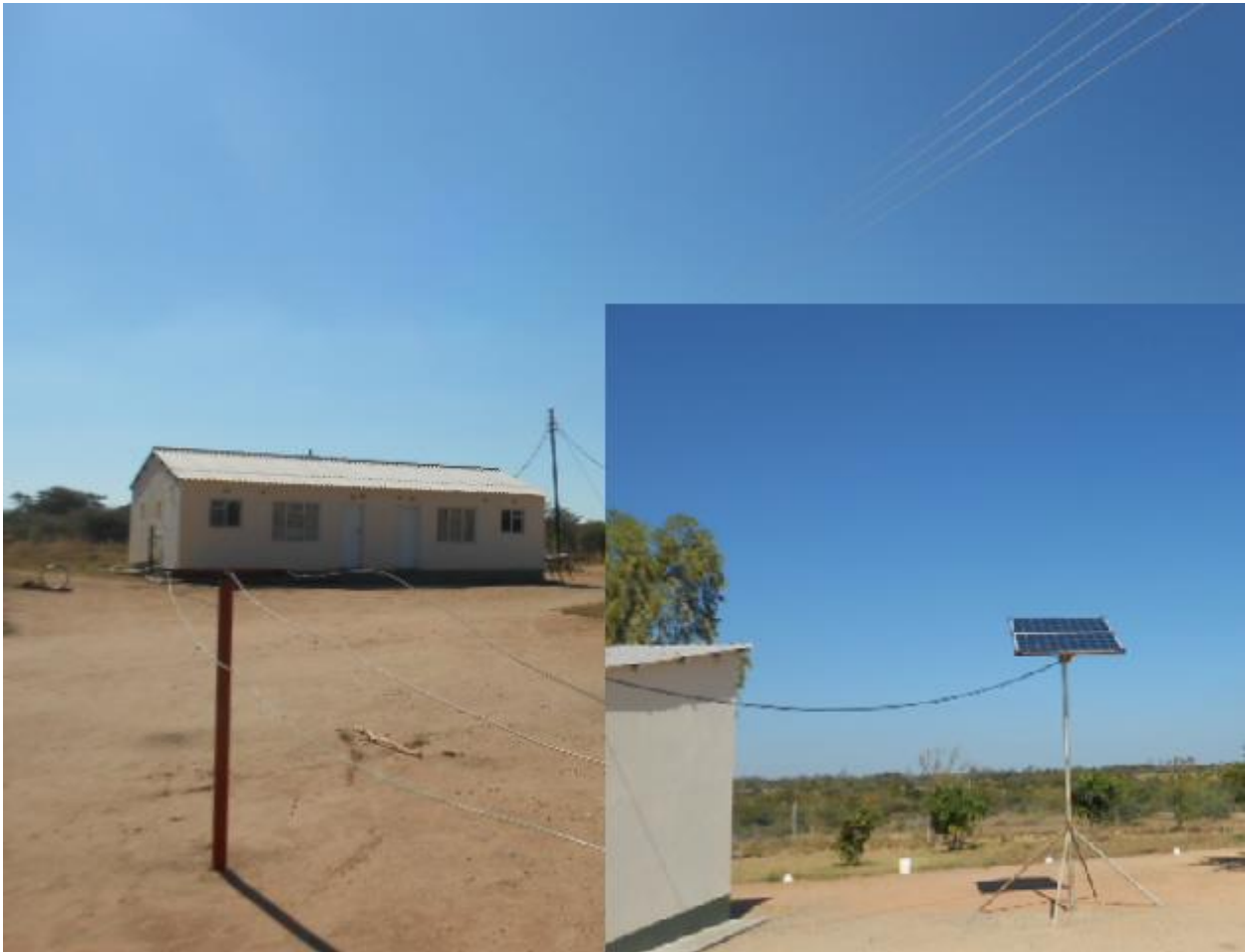
Figure 4.4 Photovoltaics system providing stand by energy for lighting in Saphila rural health centre
