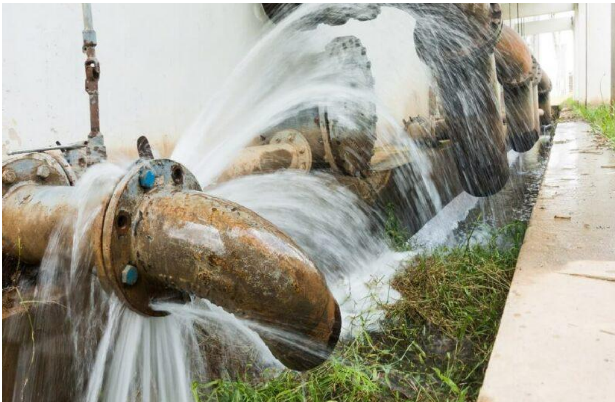
Figure 2. 2: Corroded water supply system[71]
