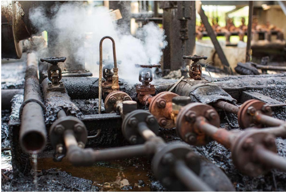
Figure 2. 5: External corrosion of oil & gas pipelines [74].
