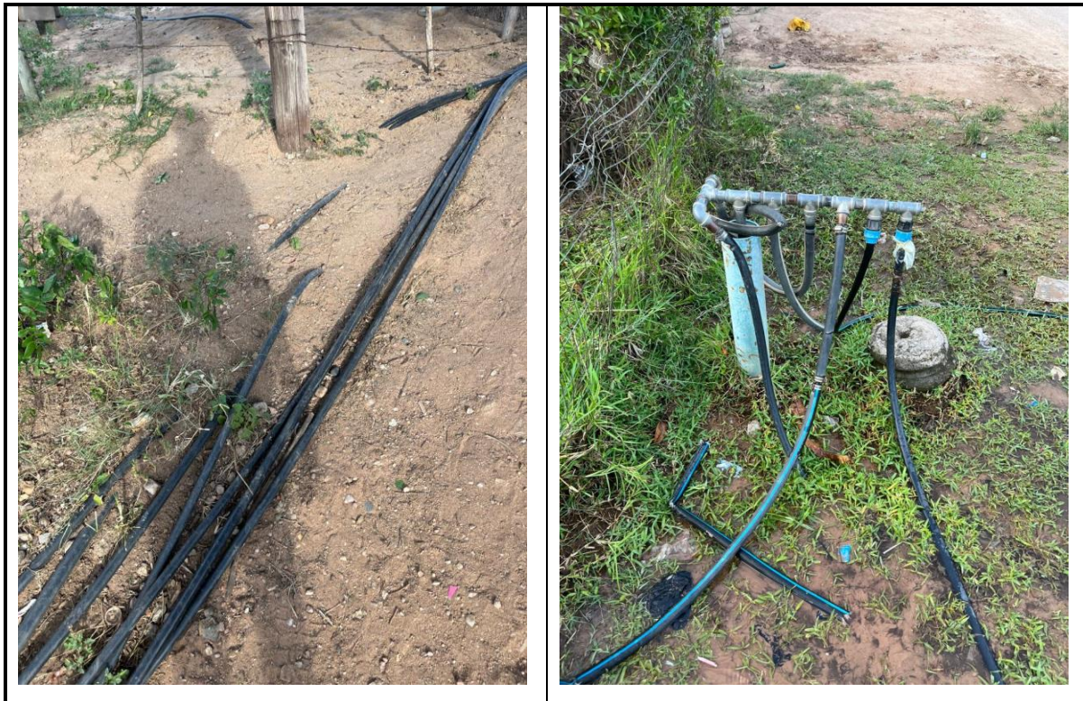
Plate 5.8: Water Infrastructure conditions
