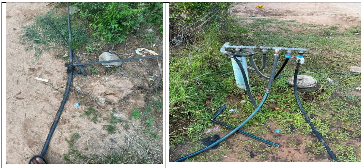
Plate 6.1: Dilapidated Water Infrastructure
