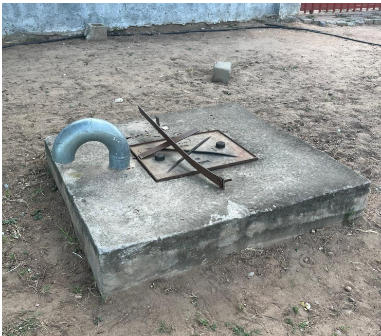
Plate 5.3: Communal Borehole Source: Author (2024).
