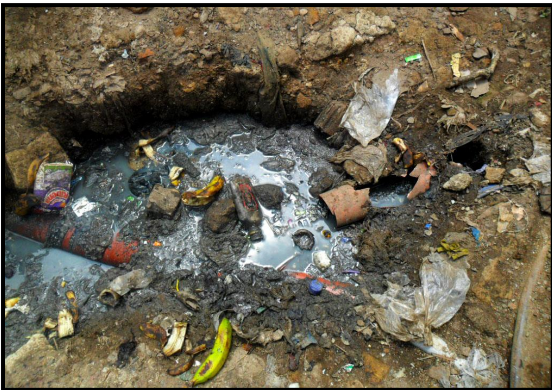
Plate 2. 9: Poor or unmaintained wastewater drainage.
