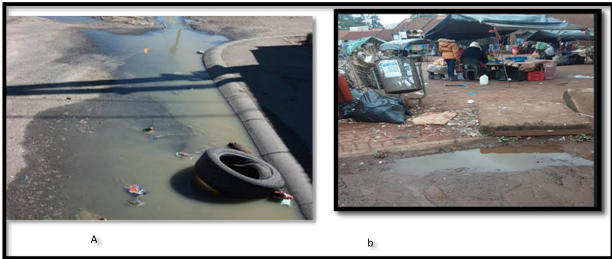
Plate 4. 2 : Blockage of water drainage
