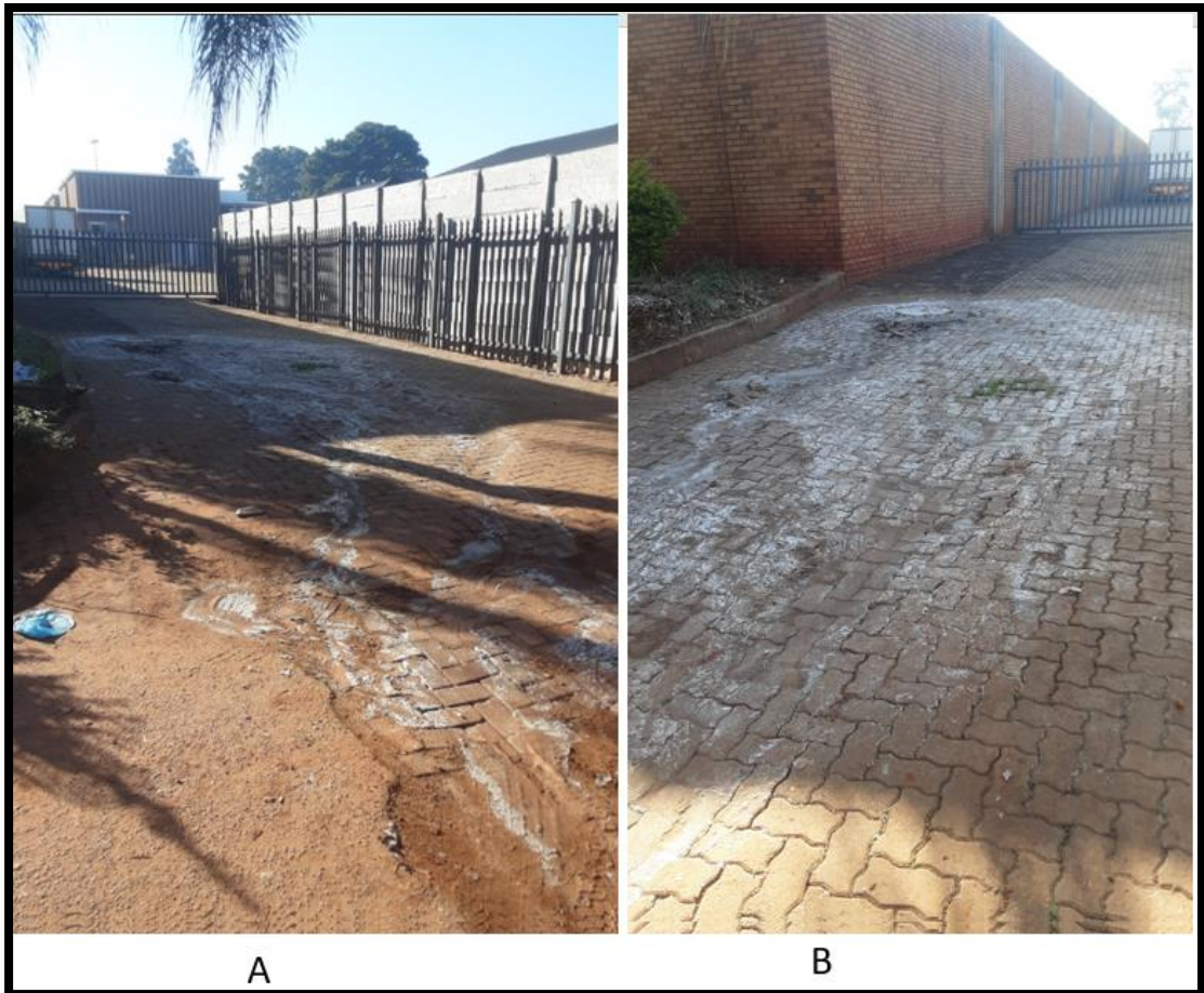
Plate 4. 1 : Spoilage sewer around street pavement in Thohoyandou CBD
