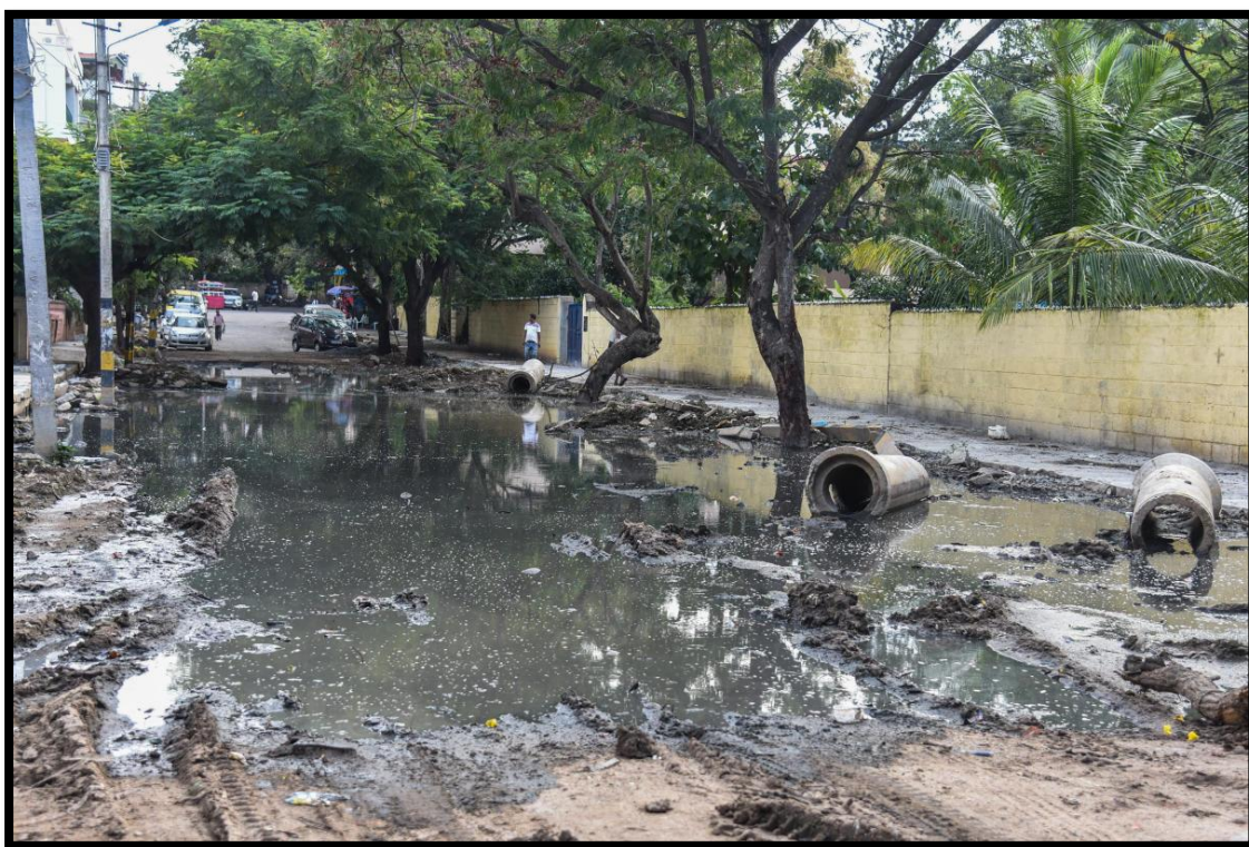
Plate 2. 3: Overflow of sewage in public spaces.
