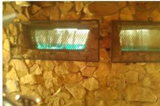
Fig: 2.3.D. View of the spring through a concrete structure with glass.
