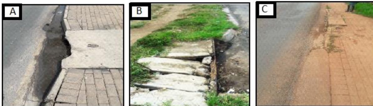
Plate 5.3: The state of roads and storm water in Thulamela, Makhado and Musina LM
