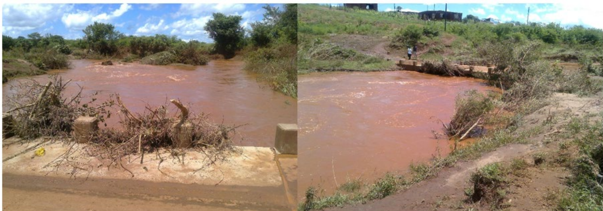
Plate 2.1: Impacts of flood on road infrastructure
