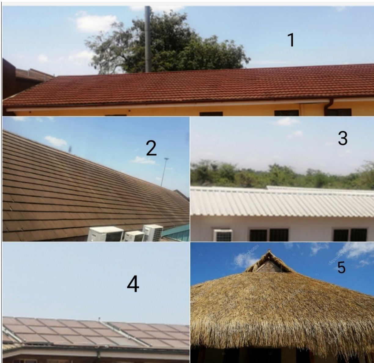
Figure 3.2: Different rooftops used to collect samples in this study, where 1 represents, Slate roofing, 2: Aluminium roofing, 3: Steel roofing, 4: Concrete tile roofing, 5: Thatched roofing
