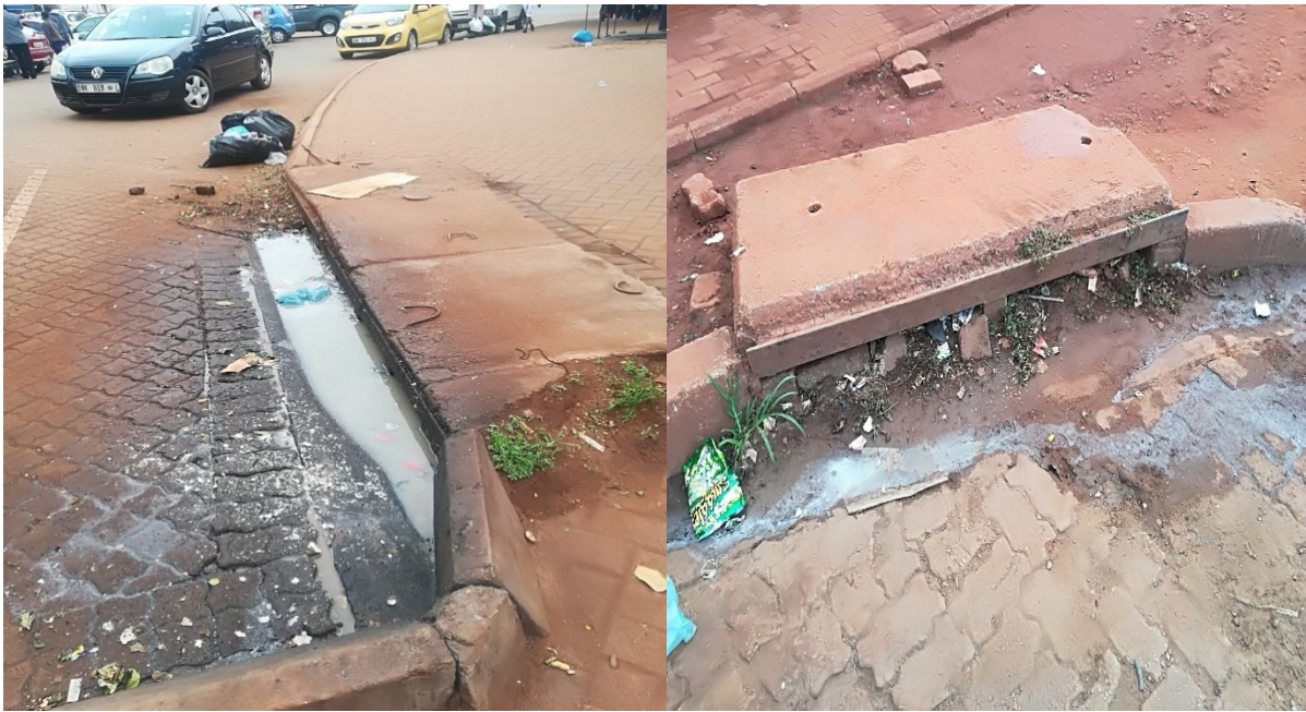
Figure 5.3: Water drainage systems blocked by food vendors' waste products in Thulamela Municipality
