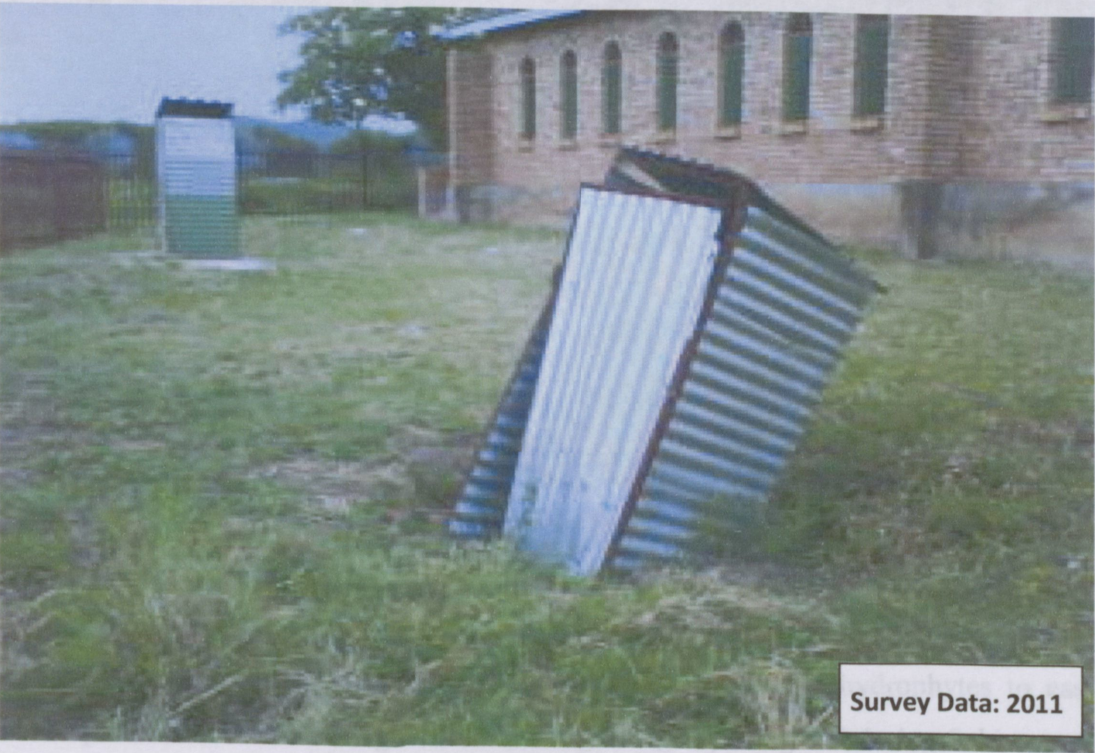
Picture 4.7 Cracked sunk toilet at Thohoyandou Block F wetland
