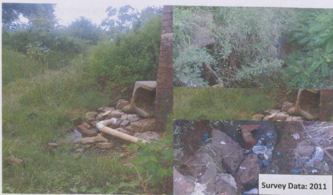
Picture 4.2: broken sewage hosepipe and deposition of waste water at Mbovana wetland
