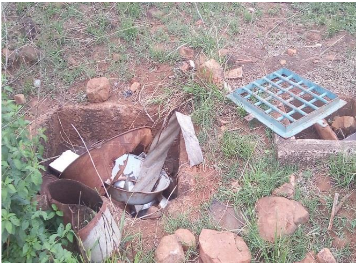
Plate 4: Broken Irrigation systems
