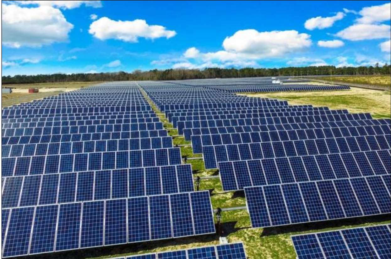
Figure 2.2: A typical solar facility (IFC, 2015).
