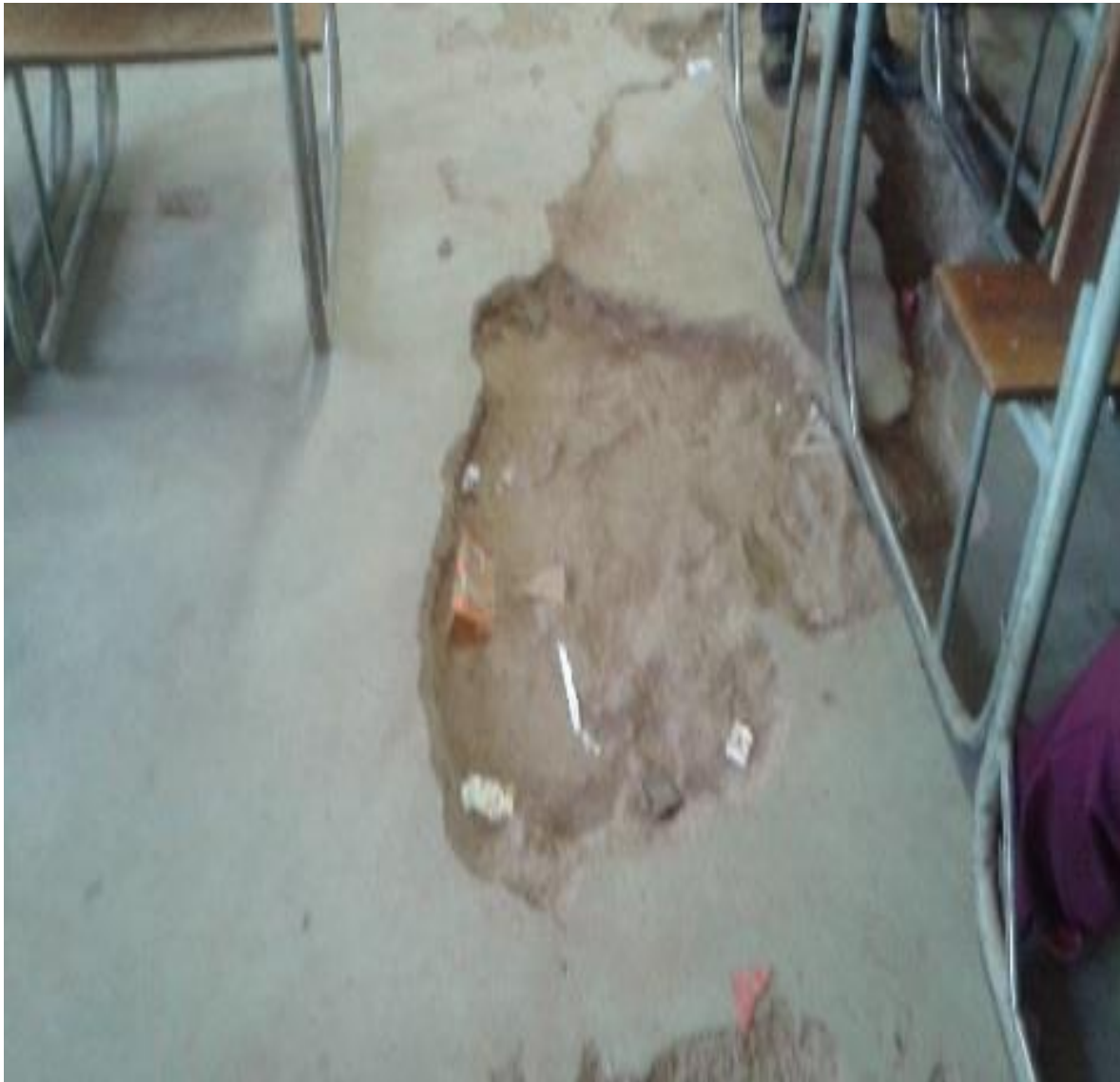
Picture 4.2: Classroom potholes
