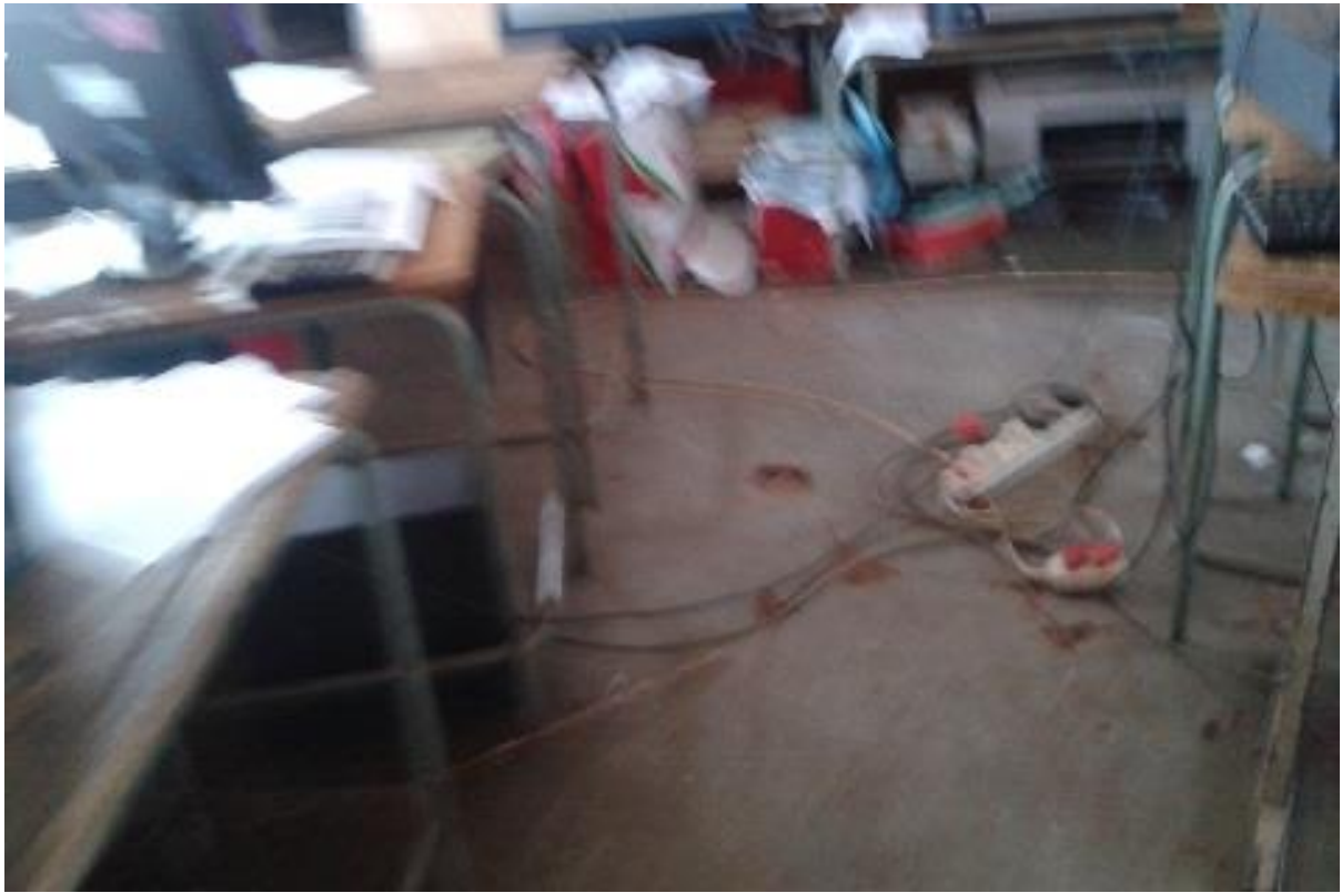
Picture 4.3: Poor electricity usage
