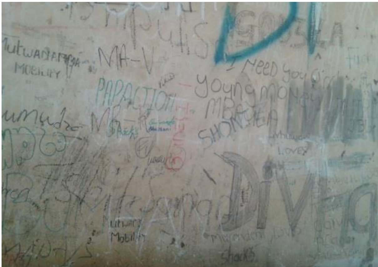
Picture 4.7: Graffiti on the walls
