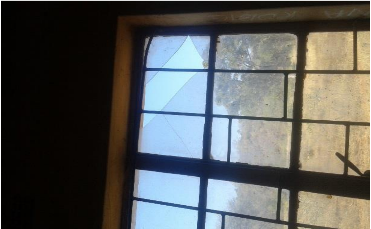
Picture 4.5: Broken windows
