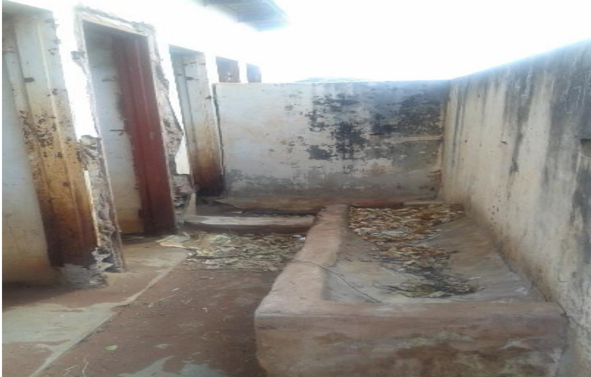
Picture 4.8: Condition of unhealthy toilets (Urinal)
