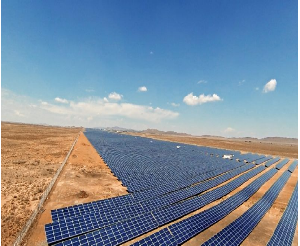
Figure 1.1: De Aar Solar Power plant in the Northern Cape Province. Source https://dearsolar.co.za/ .
