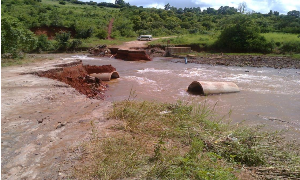
Figure 4.6: Bridge to Lwandani site damaged by flood (16/01/2013)
