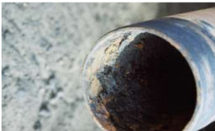
Figure 2.3: Oxygen-induced corrosion in the oil and gas pipelines [98]
