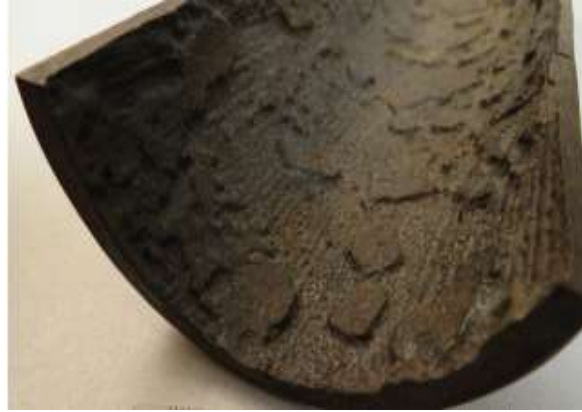
Figure 2.4: A typical example of mesa corrosion as a result of CO 2 in the pipeline [107]
