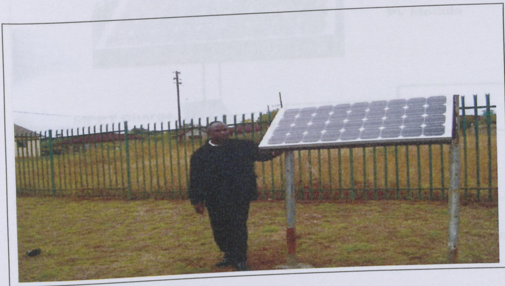
Figure 3.3. Stand alone PV module installed at the experimental site
