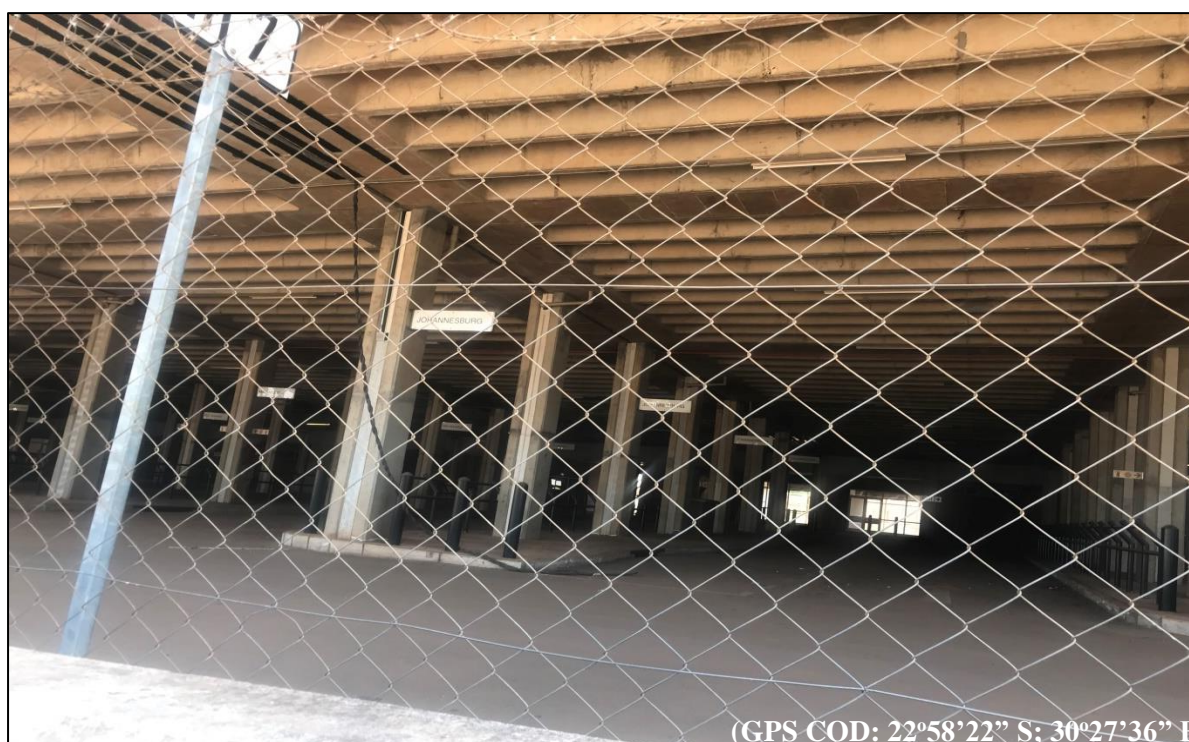
Photograph 6.4: Poorly constructed Taxi Rank Facility in Thohoyandou Town CBD
