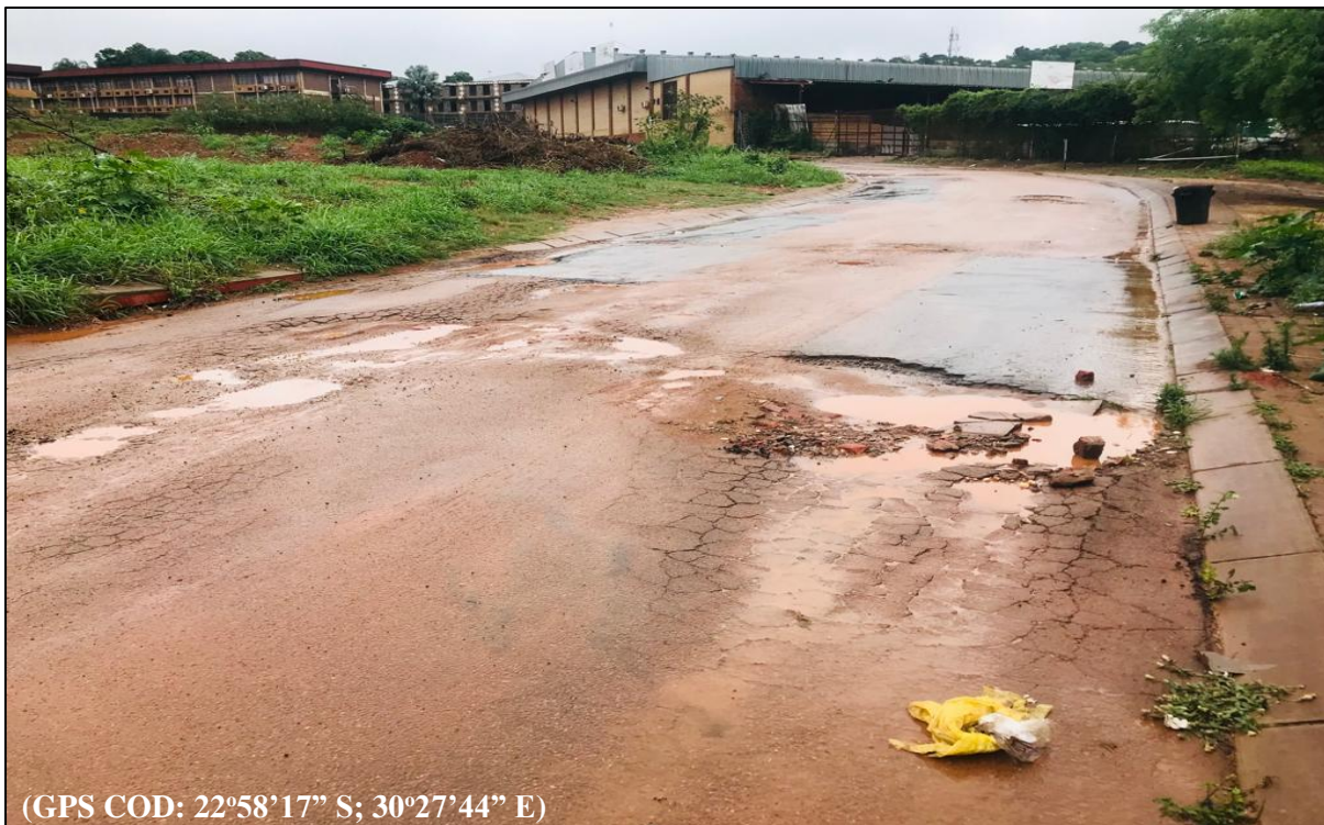
Photograph 6.6: Road/street in poor condition in Thohoyandou Town CBD Source: Author (2023)
