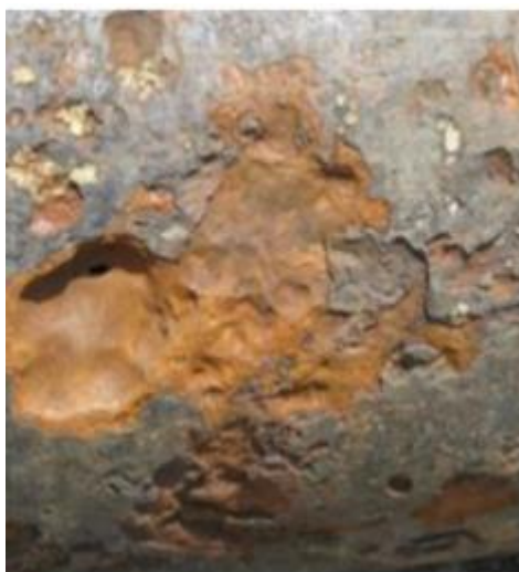
Figure 2.5: Sweet pitting corrosion on the internal lining of an oil and gas pipeline [74].
