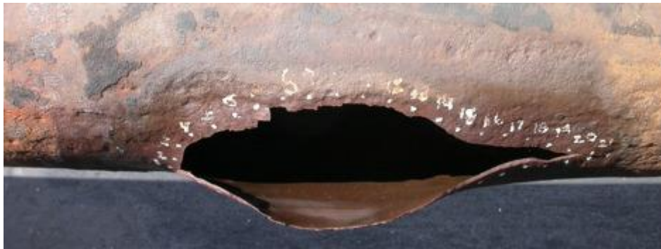
Figure 2.3: Ruptured steel pipe gradually worn out by general corrosion [58].
