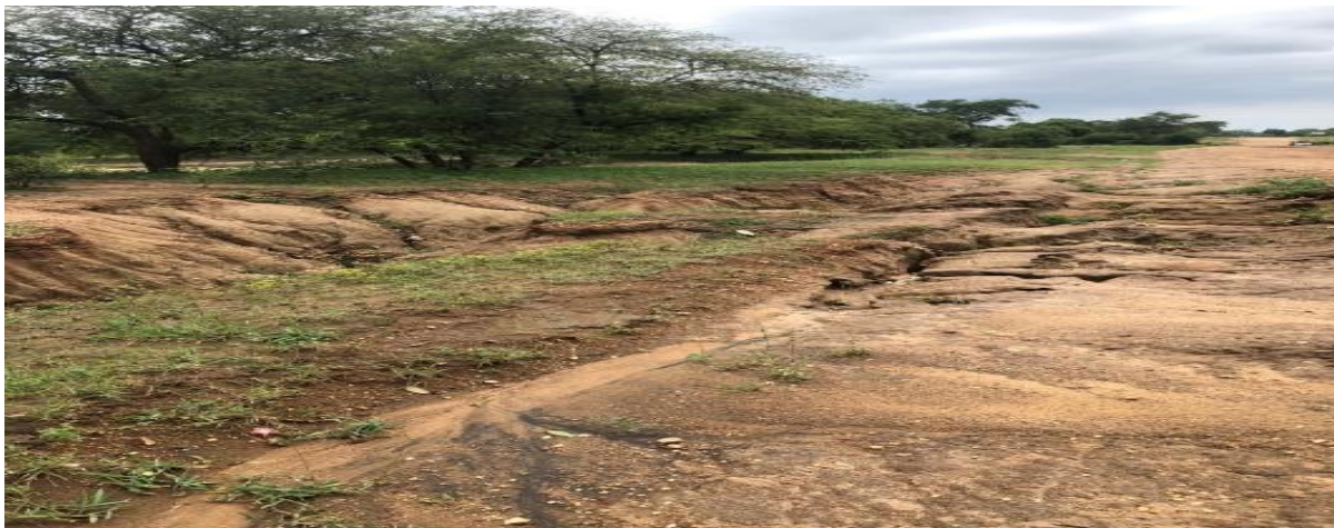
Plate 4.2: Road damage in Tsholotsho
