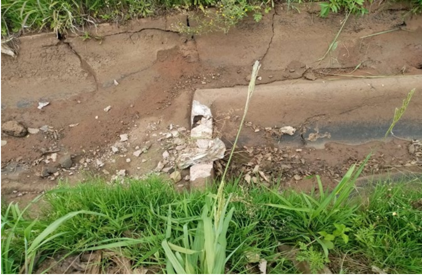
Figure 4.7: A vandalised dry main canal at Mandiwana irrigation scheme
