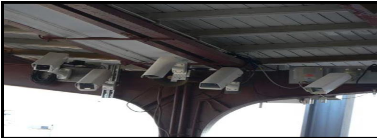
Figure 3.6. CCTV cameras for surveillance.
