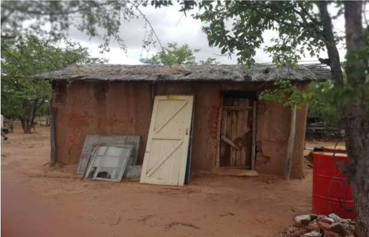
Figure 4.2: Dilapidated building in Nwanedi Nature Reserve (Survey: 2018)
