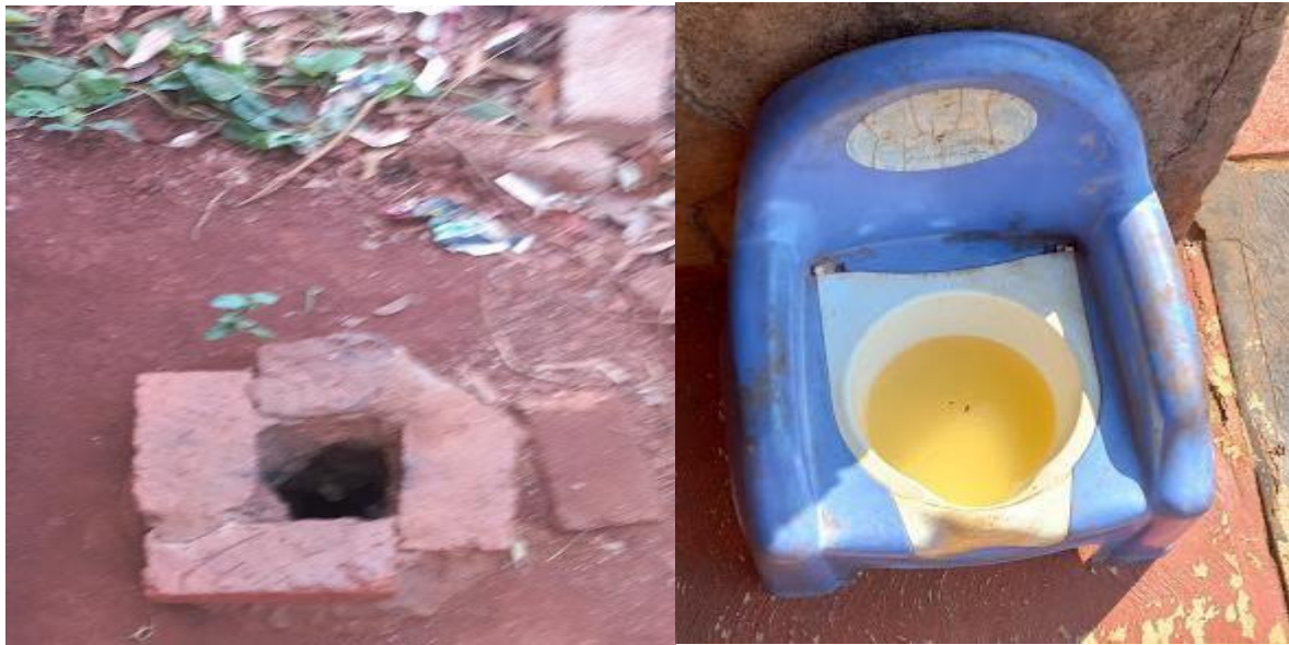
Figure 4.2: The state of the children's alternative toilets.
