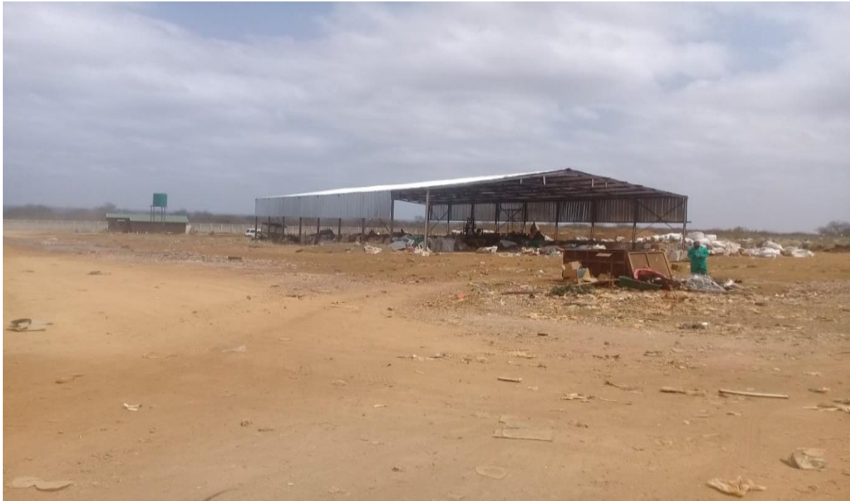
Figure 4. 17: Recycling facility at Makhado Landfill Site.
