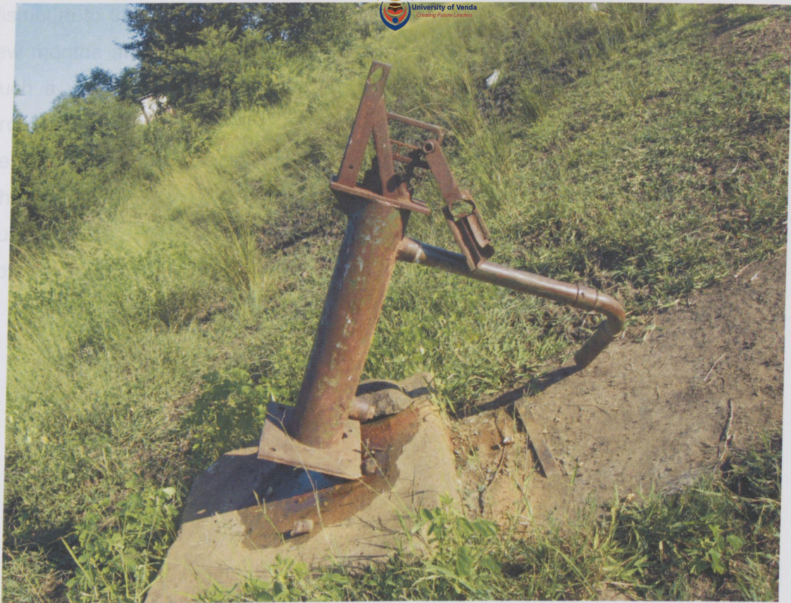
Picture 4.7: Poor maintenance of water supply system
