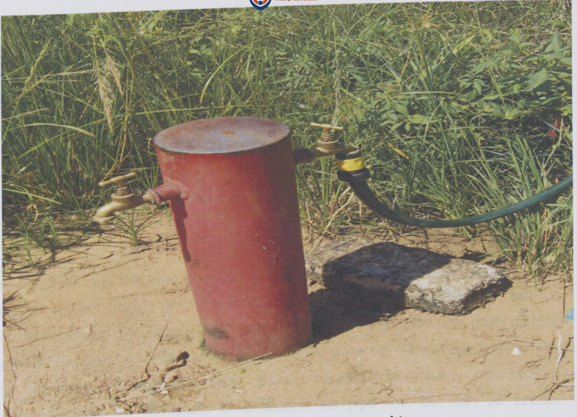
Picture 4.4: Hosepipe illegal connection to Communal tap
