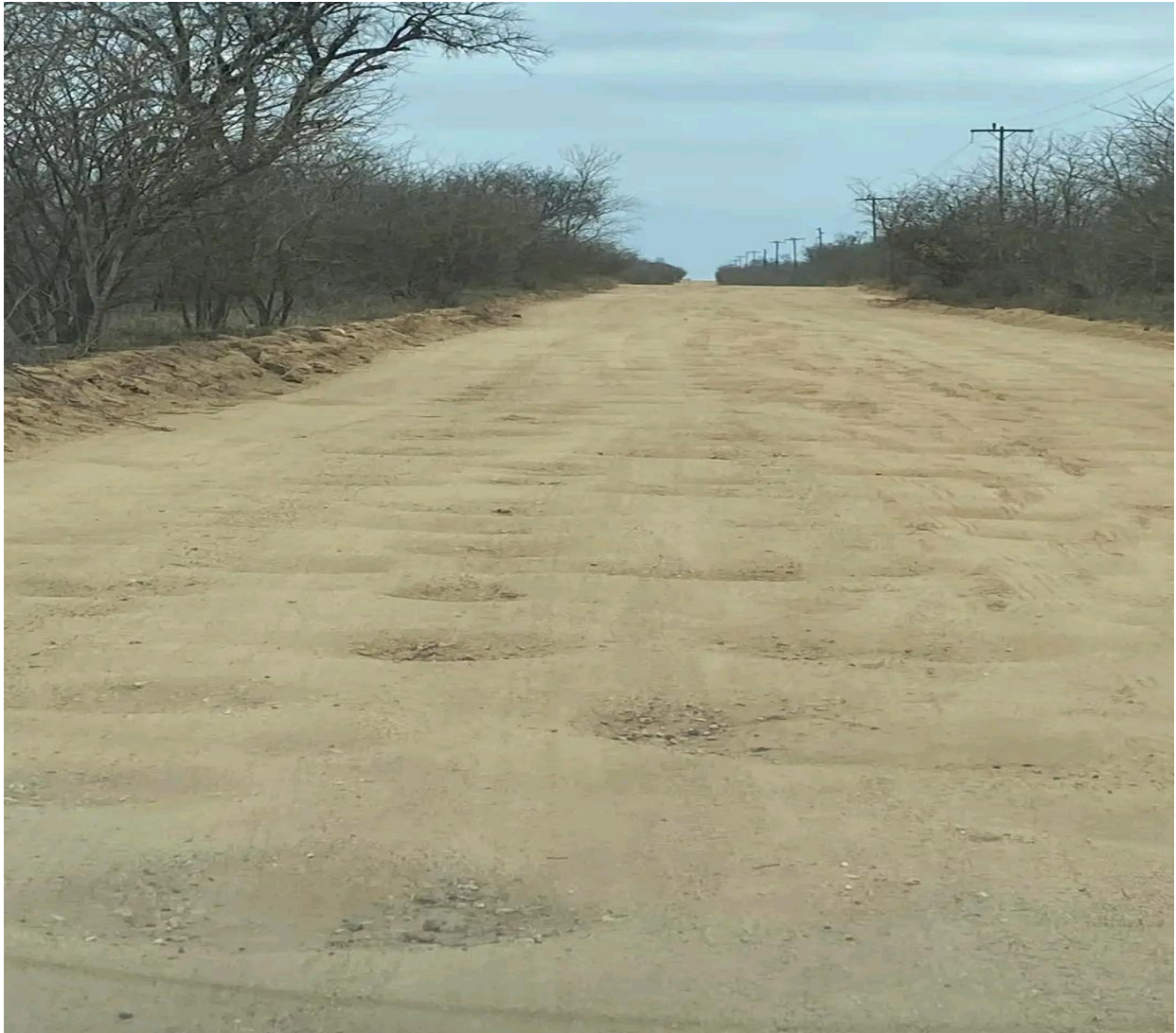
Figure 4.2: Road conditions in Tshilungoma
