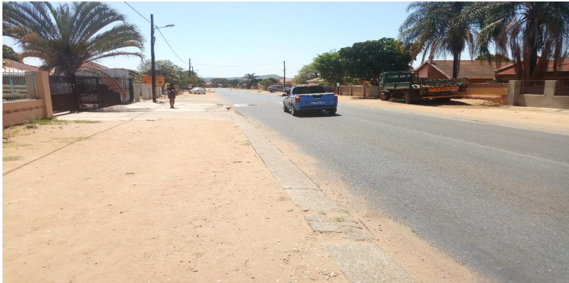
Plate 5.5: Lack of Drainage on either side of Road D 5011 at Section B, Nkowankowa (Source: Author's Field Photo, 2018)
