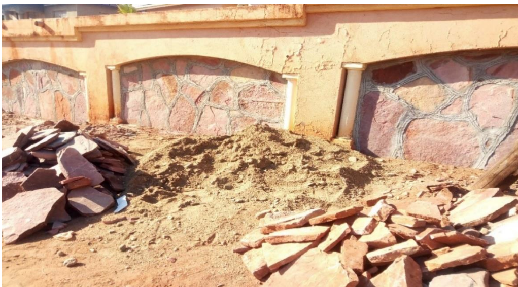
Plate 7.9: A typical house reinforced with stones and concrete in Hoedspruit (Source: Author's Field Data, 2019)
