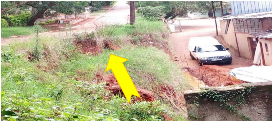
Plate 5.6: Road under threats by runoff occasioned by steep terrain and lack of Drainage in Modjadjiskloof (Source: Author's Field Data, 2019)
