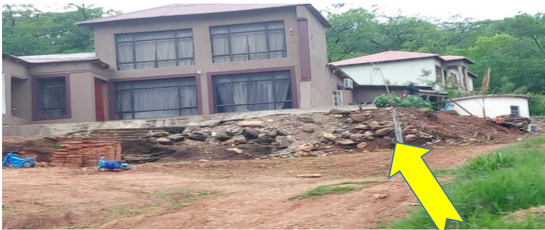
Plate 5.7: Building Foundation threatened by steep slope-enhanced erosion in ModjadjisKloof (Source: Author's Field Data, 2019)
