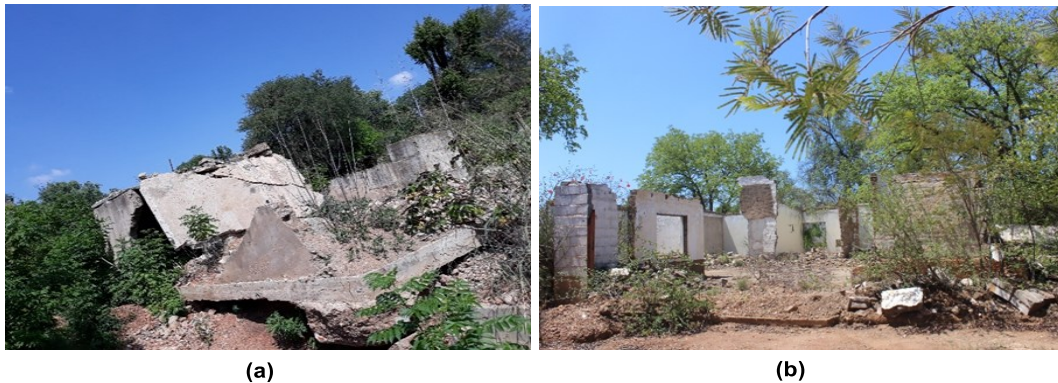
Figure 4. 6: The collapsed (a) and (b) standing dilapidated buildings in abandoned mine sites
