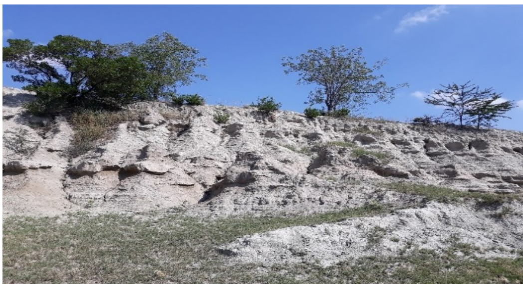
Figure 4. 4: The evidence of devastating effect of erosion on the slopes of the tailings dumps of Louis Moore
