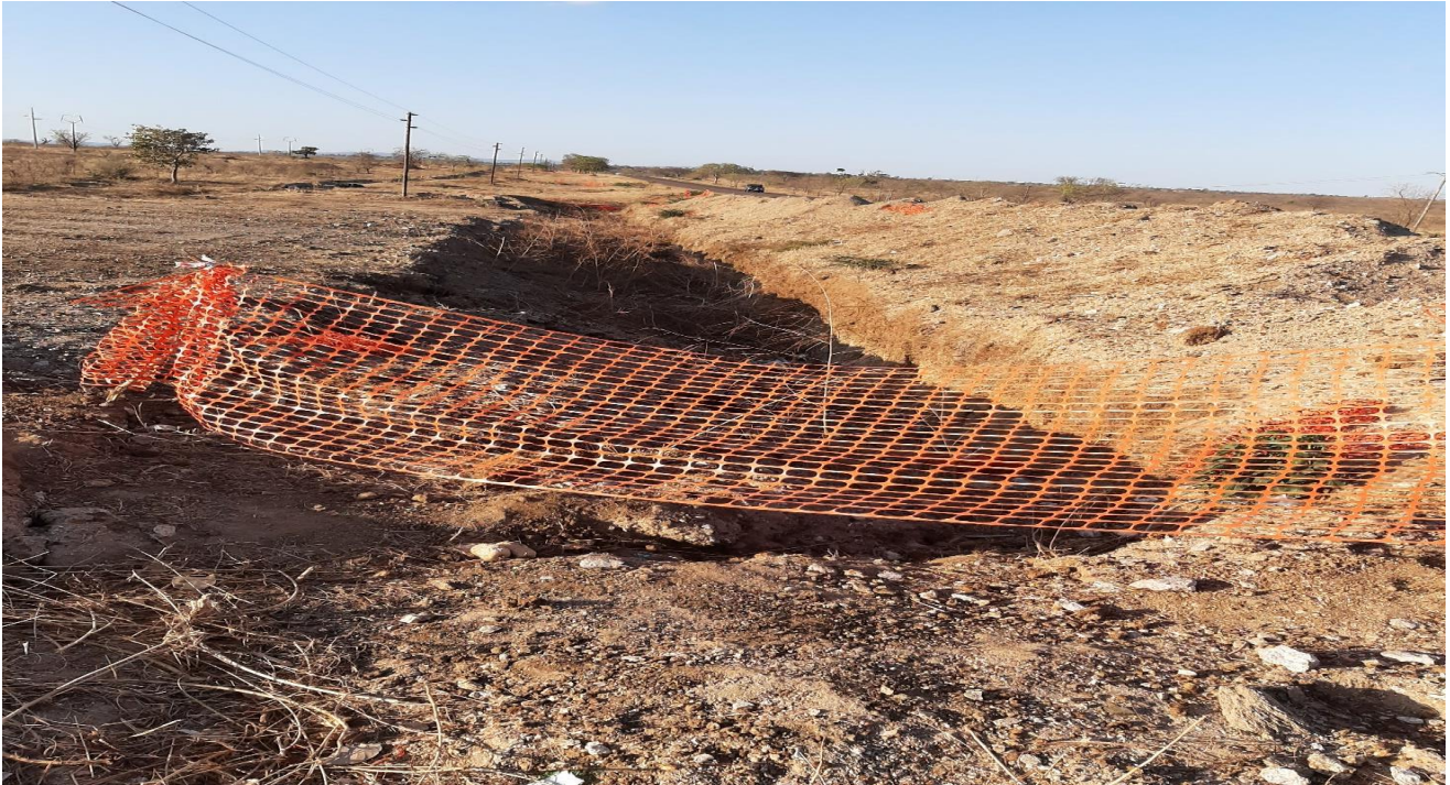
Figure 6.7: Trenches of water pipelines left unattended
