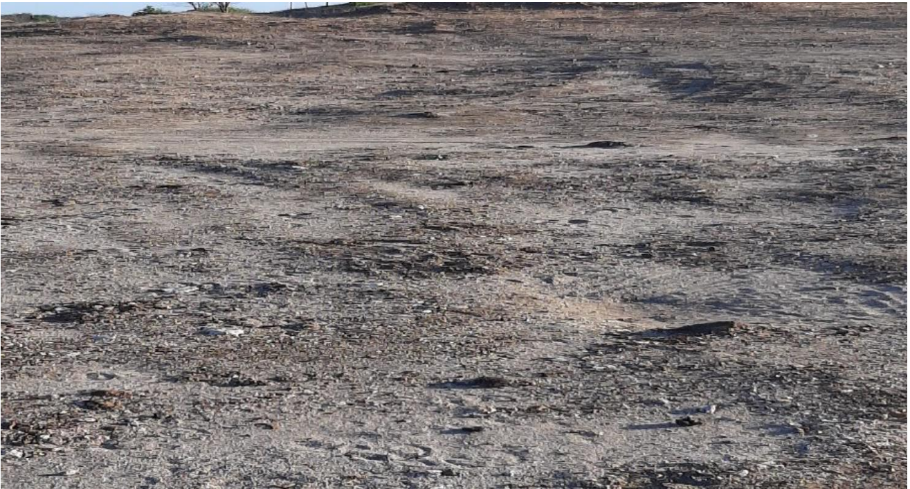
Figure 6.8: Incorrect water pipeline installed
