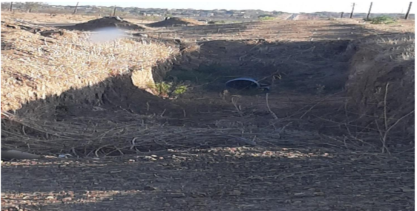
Figure 6.5: Incomplete water pipeline next to Zinja Lodge
