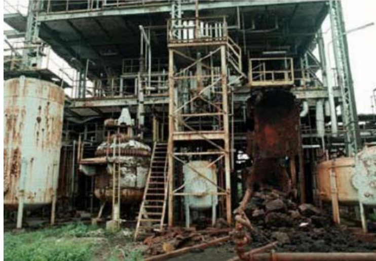
Figure 2.25: 1984 India chemical plant after exploding [132].
