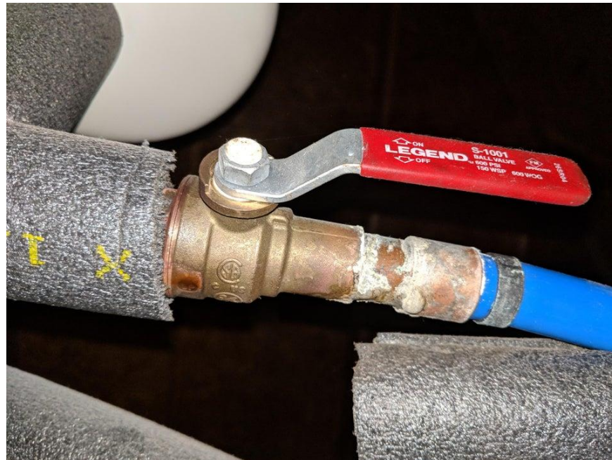
Figure 2.16: An example of selective corrosion.
