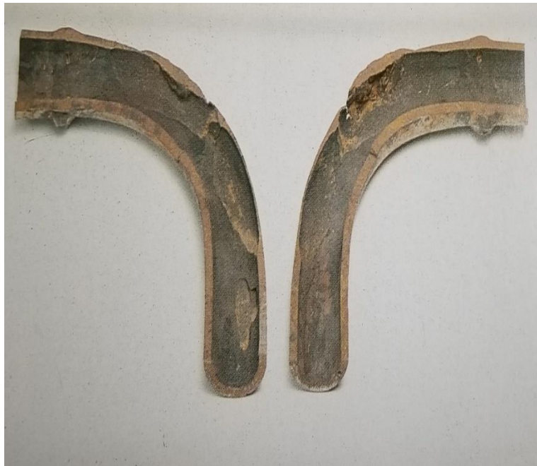
Figure 2.14: The failure at a pipe elbow due to erosion-corrosion [82].
