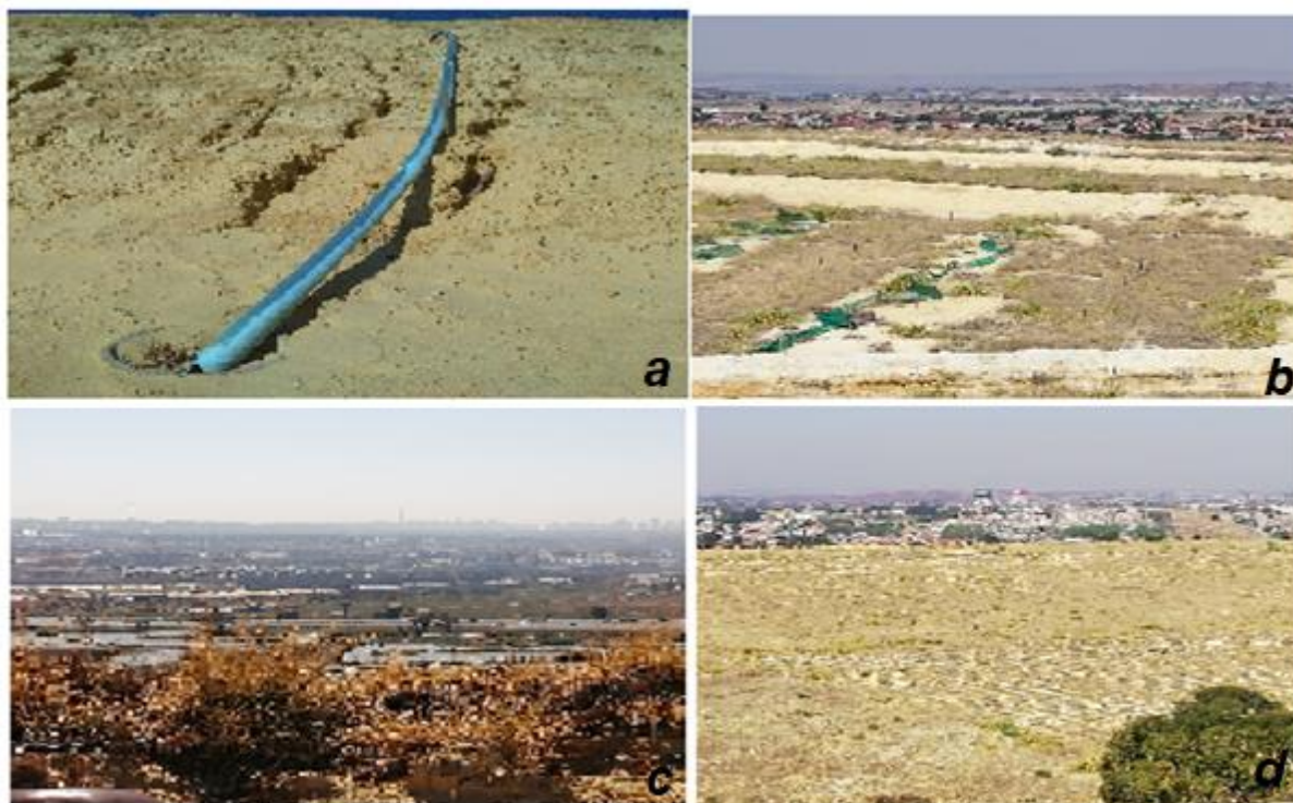
Figure 3.2: Rehabilitation and retention of the leachate activities, a drainage pipe, b dust control, c leachate retention ponds and d vegetation cover.
