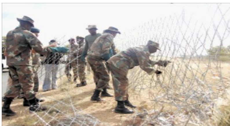
Figure 5: Members of the SANDF effecting basic repairs on the South Africa-Zimbabwe border fence.
