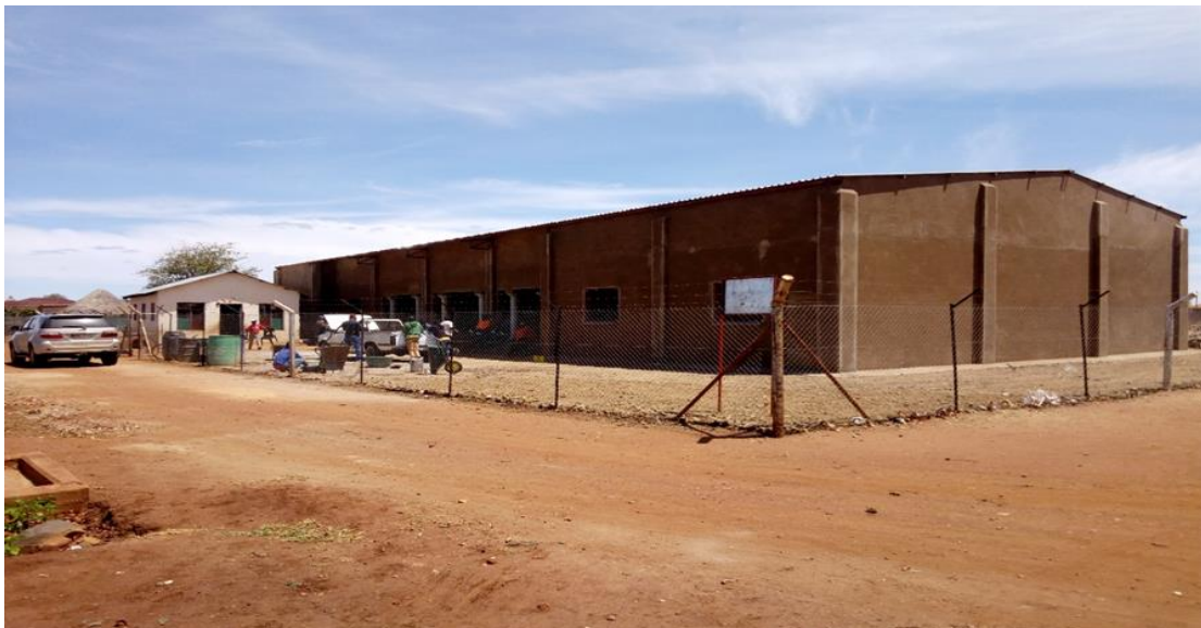
Ongoing construction of Creche (next to a community hall) at Mabilingwe village
