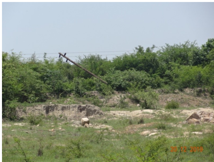
Figure 4.11: Electricity power line damage by mining operation
