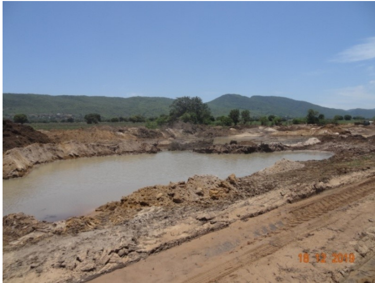
Figure 4.7: Excavation filled with groundwater
