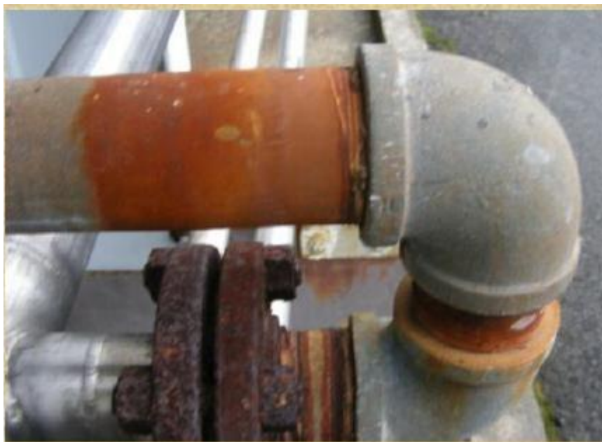
Figure 2. 1: Galvanic corrosion of steel pipe connected to copper connector 33
