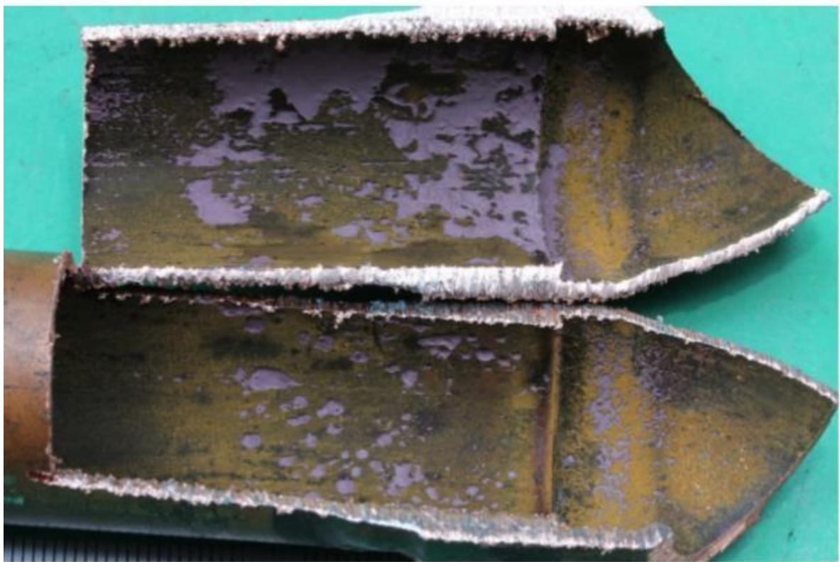
Figure 2. 2: Erosion corrosion inside the pipe 33 .
