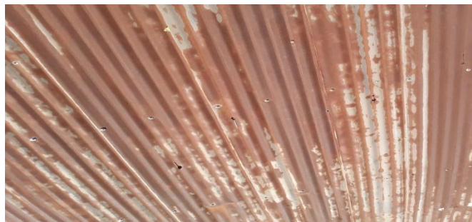
Figure 1.1: Corroded hot-dip galvanised corrugated steel sheet used for roofing purpose.
