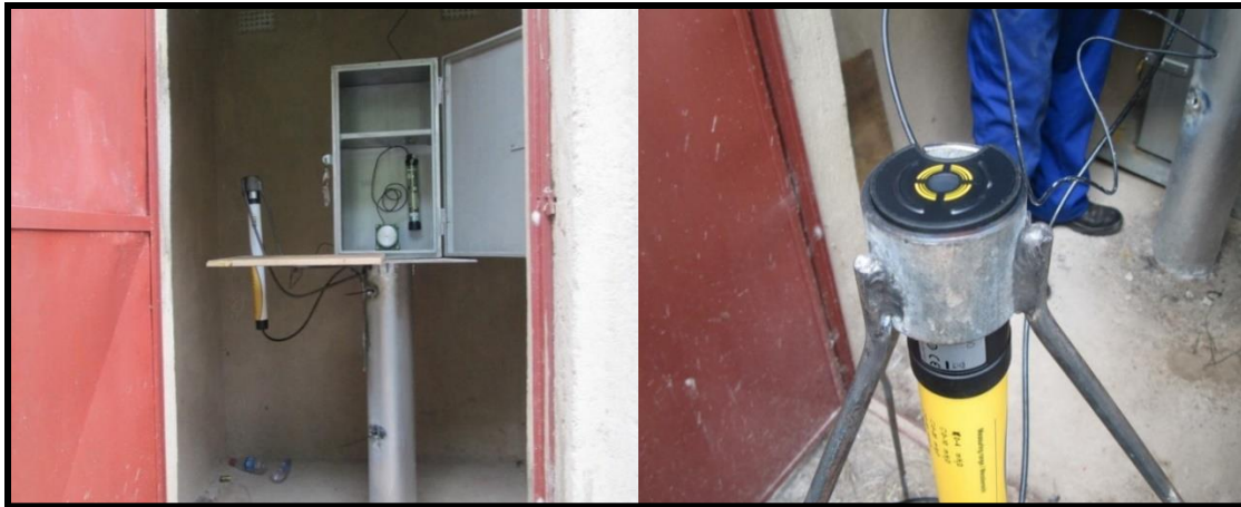
Figure 5. 3: Pictures of the automated data loggers that have been installed at the flow gauging stations the Pungwe River on the Zimbabwean side. From Left, Ecolog500 data logger at F22 and to the right, Thalimed data logger for F24.
