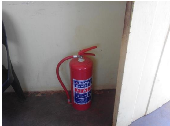
Plate 5-7: fire extinguisher that is located at the site office
