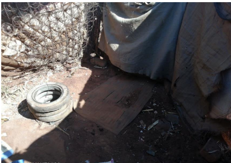
Photograph 5.3. Inside a pit latrine in Hlophekane Informal Settlement
