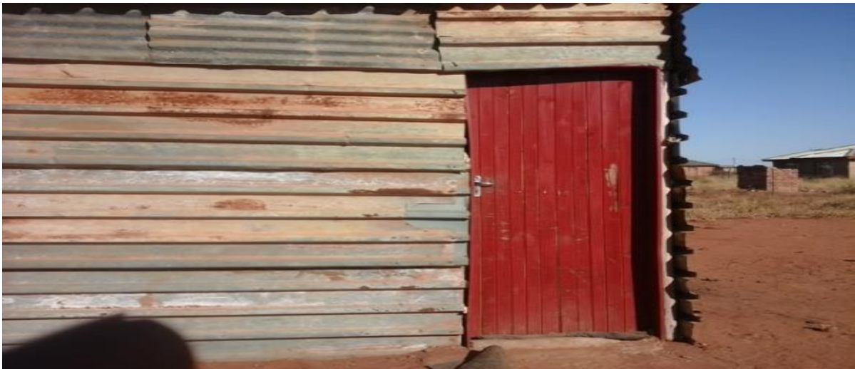
Figure 4.3: No fence nor gate around the shack
