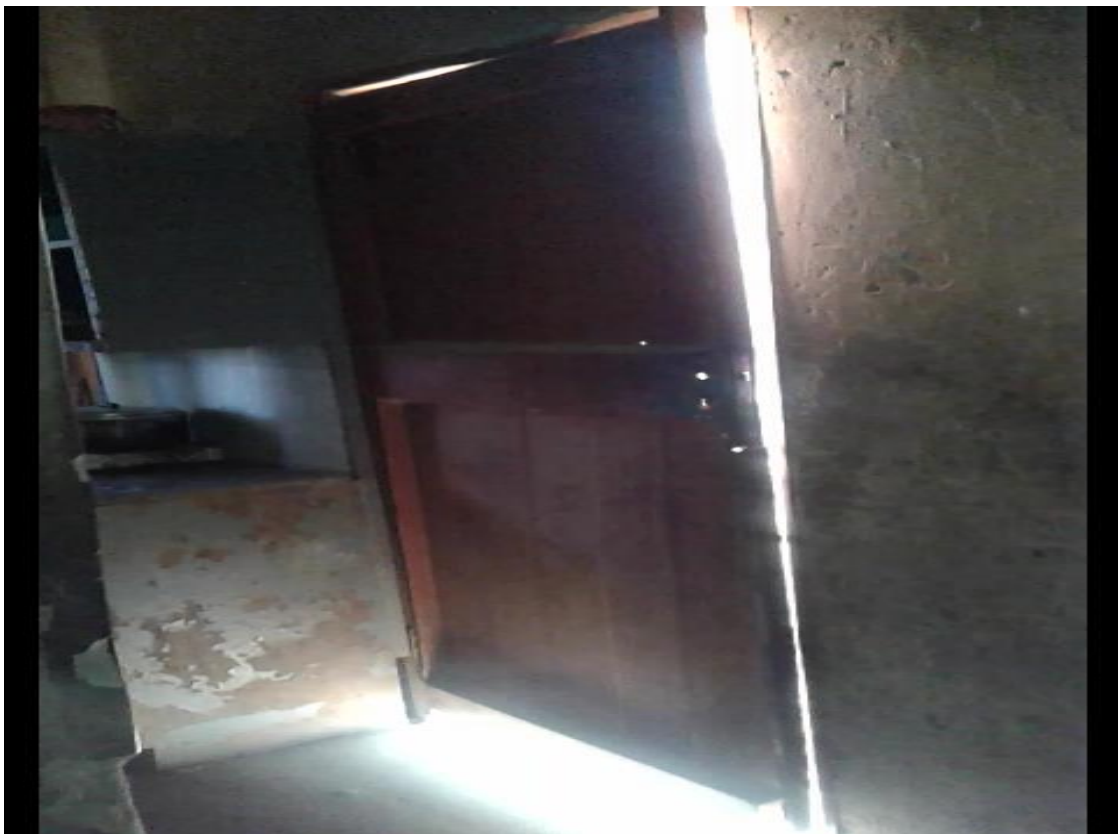
Figure 4.2: Poor state of the door
