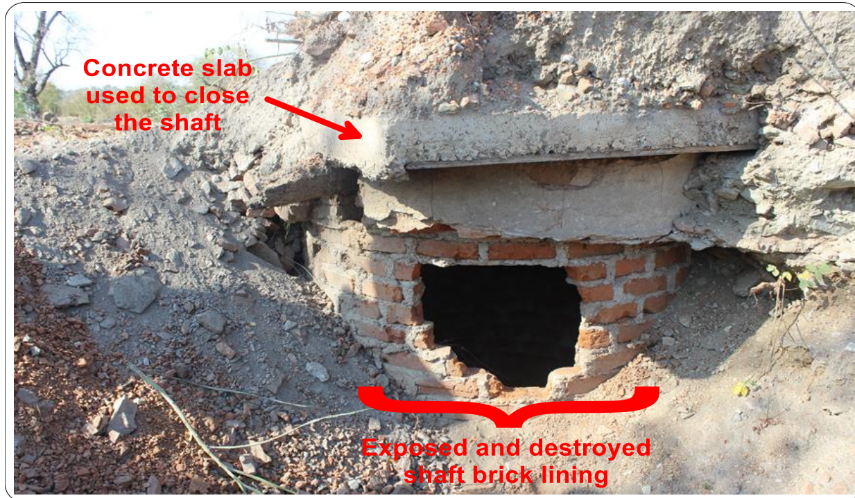
Figure 4.4: An illustration of the shaft lining destroyed by illegal miners.
