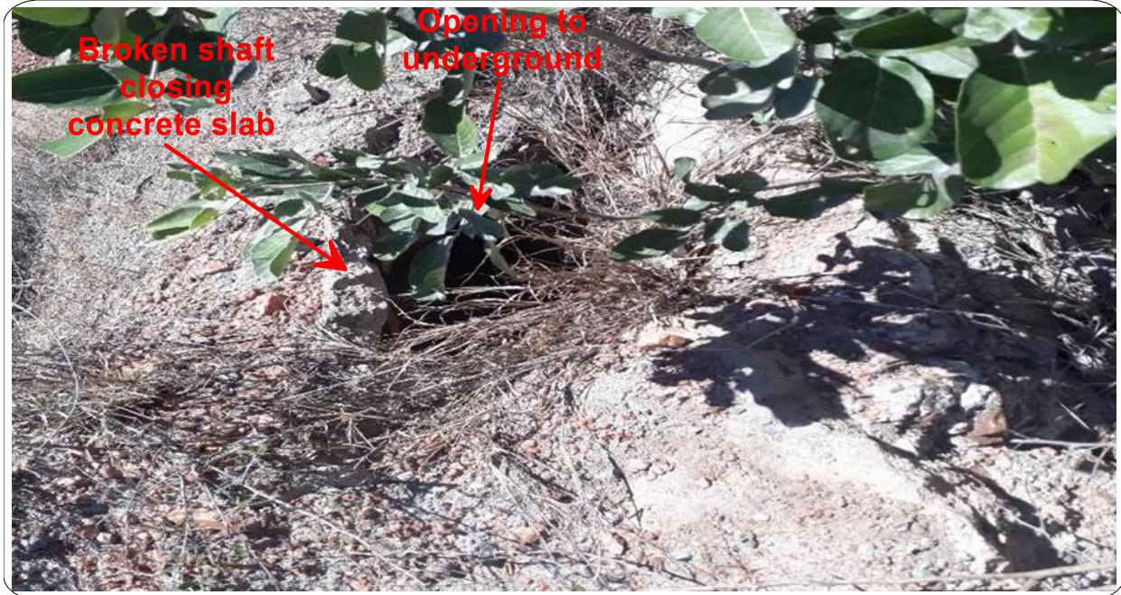
Figure 4.3: An illustration of the shaft covered with a deteriorated concrete slab and timber platform at Louis Moore Mine.
