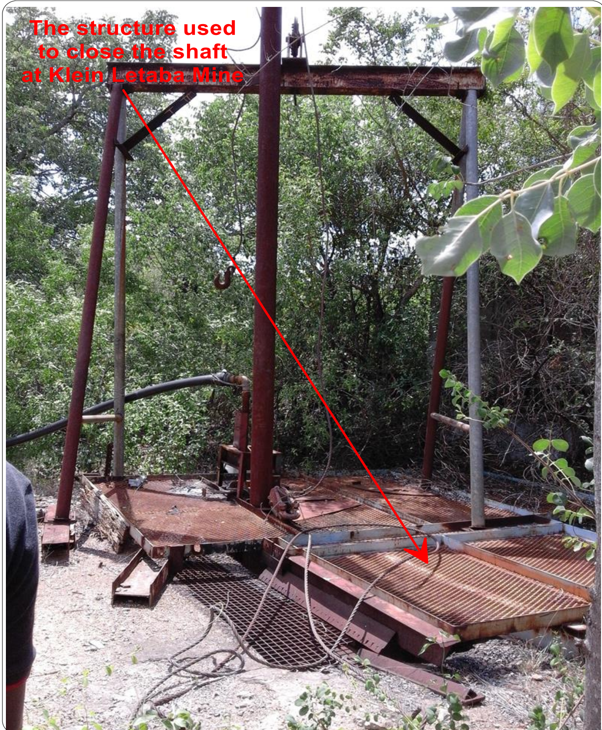
Figure 4.5: An illustration of mine shaft closed with steel structure at Klein Letaba.
