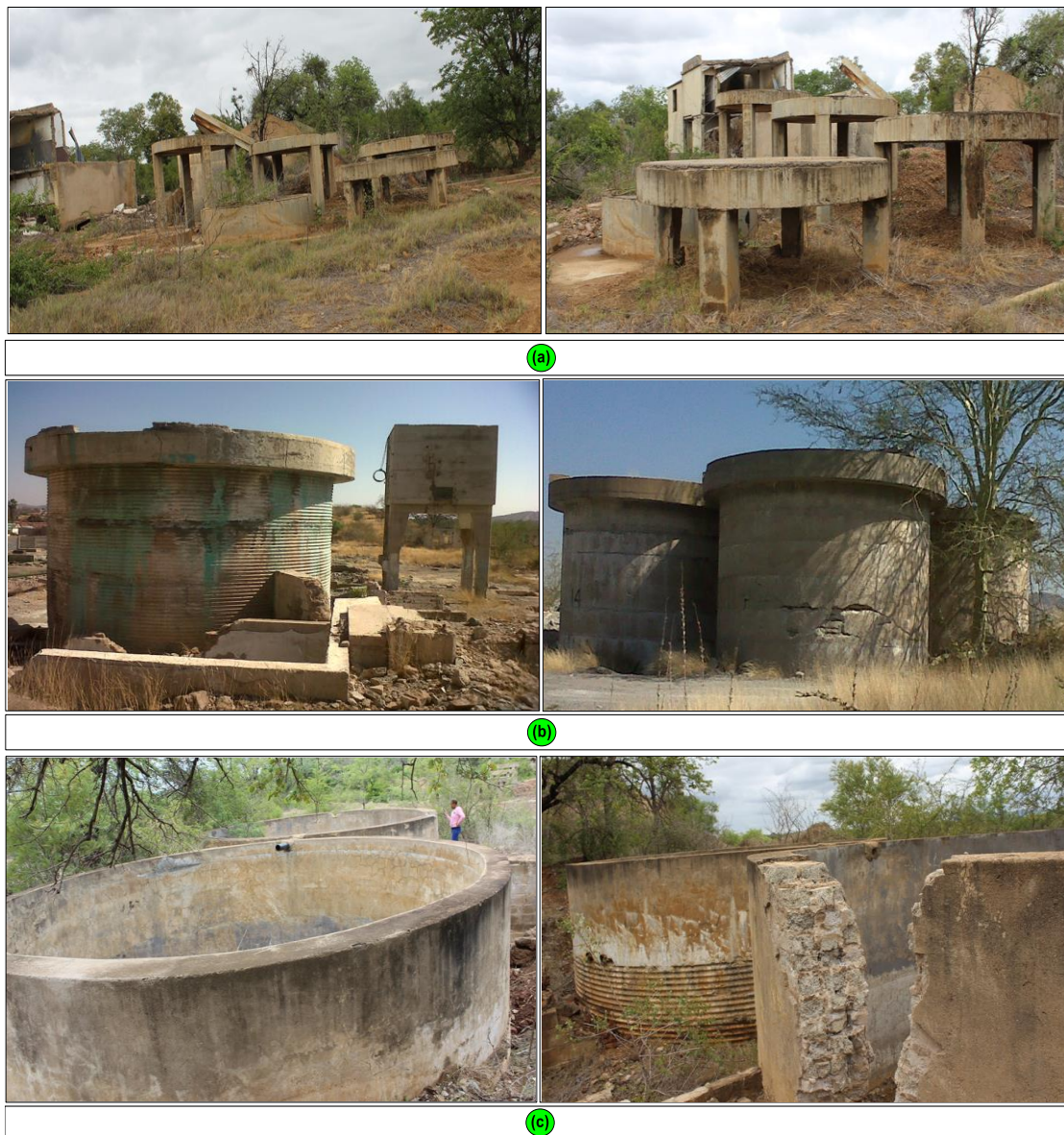
Figure 5.11: An illustration of the mounting stands and water reservoirs found at different parts of abandoned mine sites in the study area.
