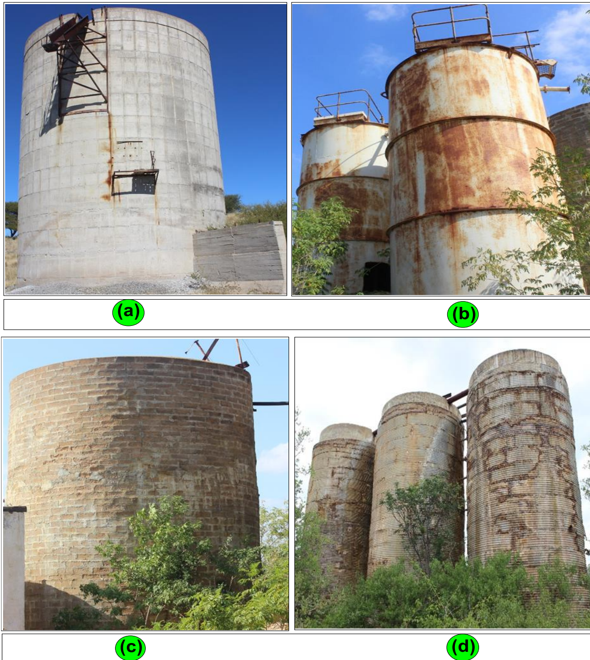
Figure 5.2: An illustration of the abandoned tall cylindrical structures in the study area. (a) reinforced concrete silo, (b) steel made agitation tanks, (c) cement bricks made ore-bin, and (d) zinc protected plastered cement bricks silos.
