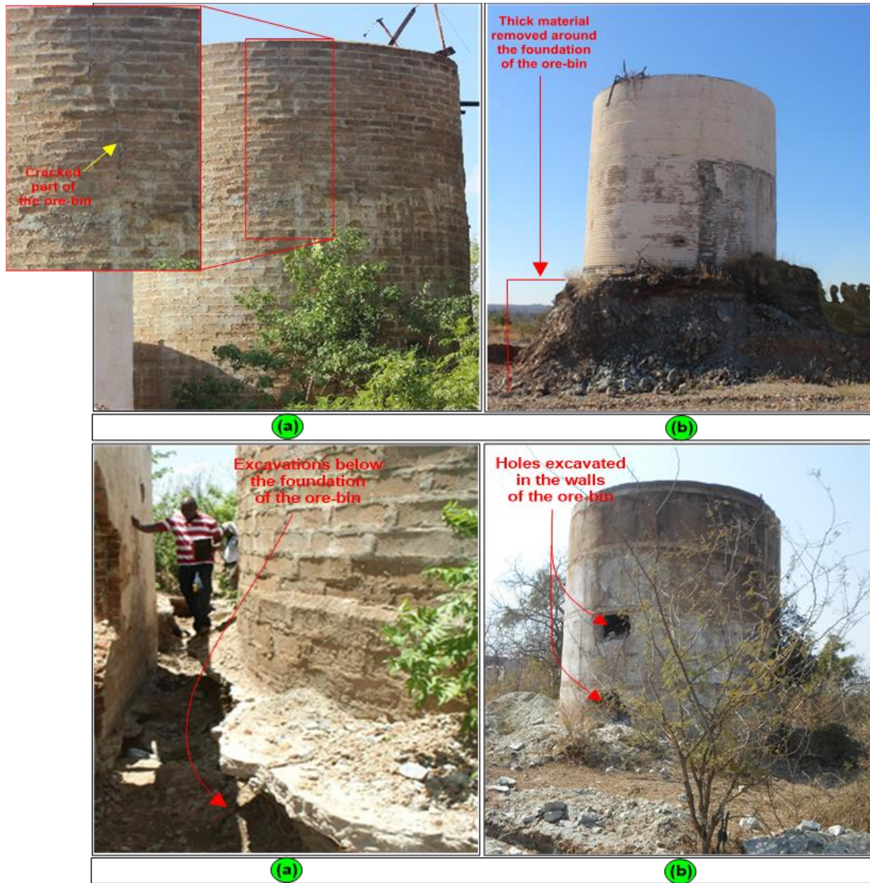
Figure 5.3: An illustration of the state of the unstable abandoned cylindrical structures in the study area.
