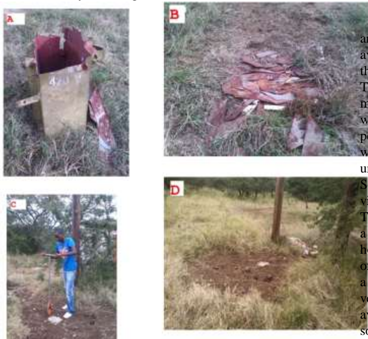
Fig 4: (A) The vandalized transfer that was damaged by the thieves, (B) the contents of transformer were thrown into the ground, (C) collecting of samples from the contaminated site and (D) notice there is no grass growing at the contaminated site
