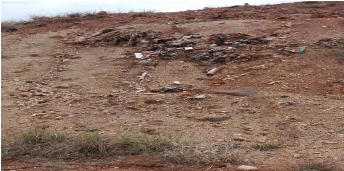
Figure 4.13: Soil erosion on rehabilitated cell
