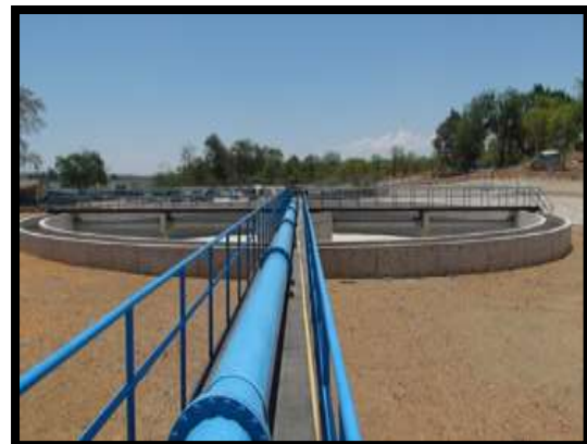
(b) Beitbridge water treatment facility
